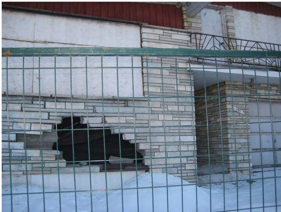
Photograph 6: View of the Site building and the wall damage on the façade.
