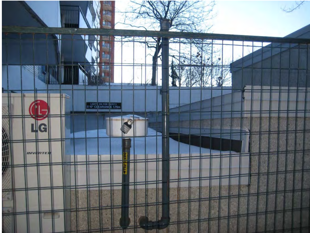
Photograph 5: View of the fill and vent pipes noted on the adjacent apartment building complex to the south.
