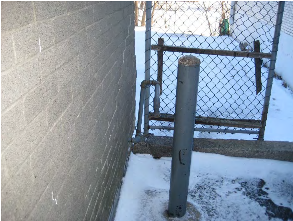
Photograph 8: View of the disconnected natural gas piping previously supplying gas to the house.
