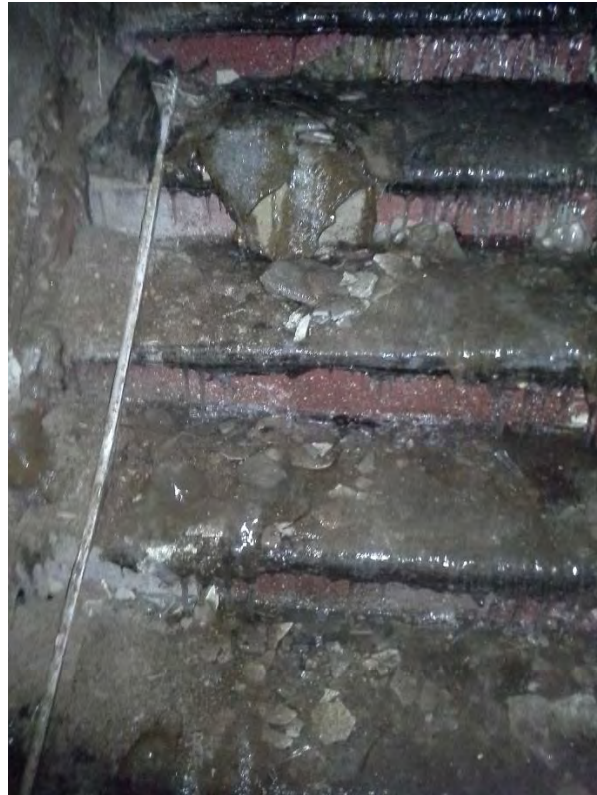
Photograph 9: View of the ice covered stairs in the house.
