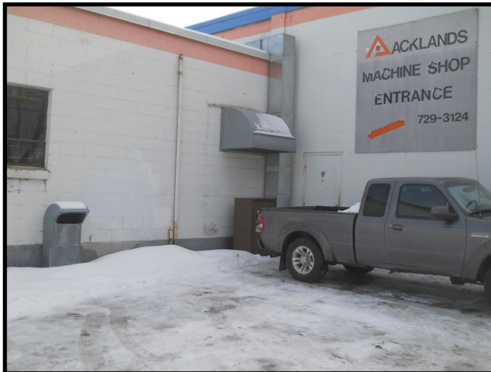
Photograph 4: View of the vent and fill pipes to the northwest of the automotive garage. View is looking southeast.
