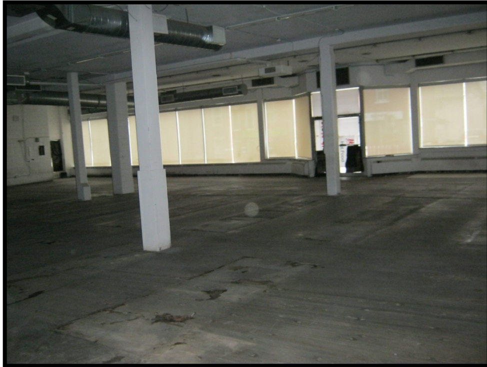
Photograph 7: View of the interior of the ground floor of the vacant commercial (north) portion of the subject building. View is looking northwest.
