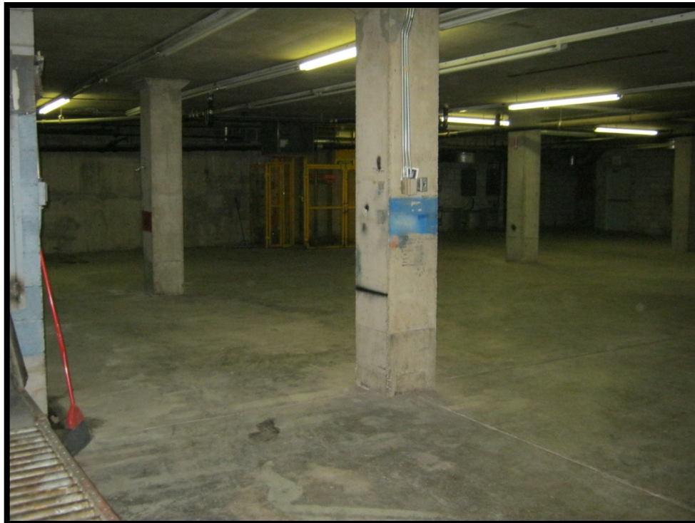
Photograph 8: View of the interior of the basement of the vacant commercial portion of the subject building, looking northeast.
