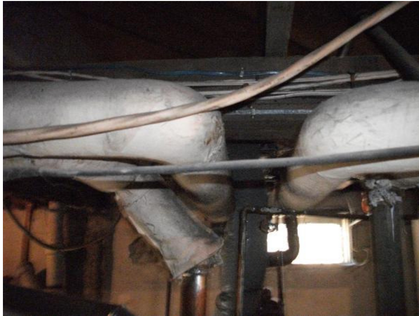
Photograph 7: Potential asbestos-containing pipe elbows in basement of 99 Norman Street.
