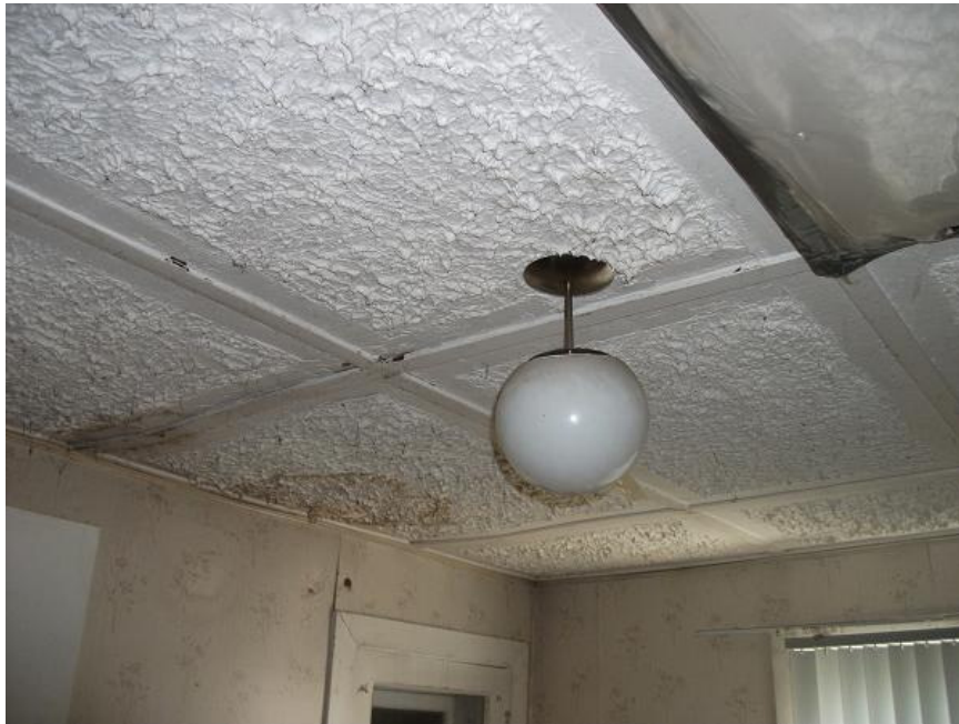
Photograph 8: Potential asbestos-containing plaster ceiling at 105 Norman Street.
