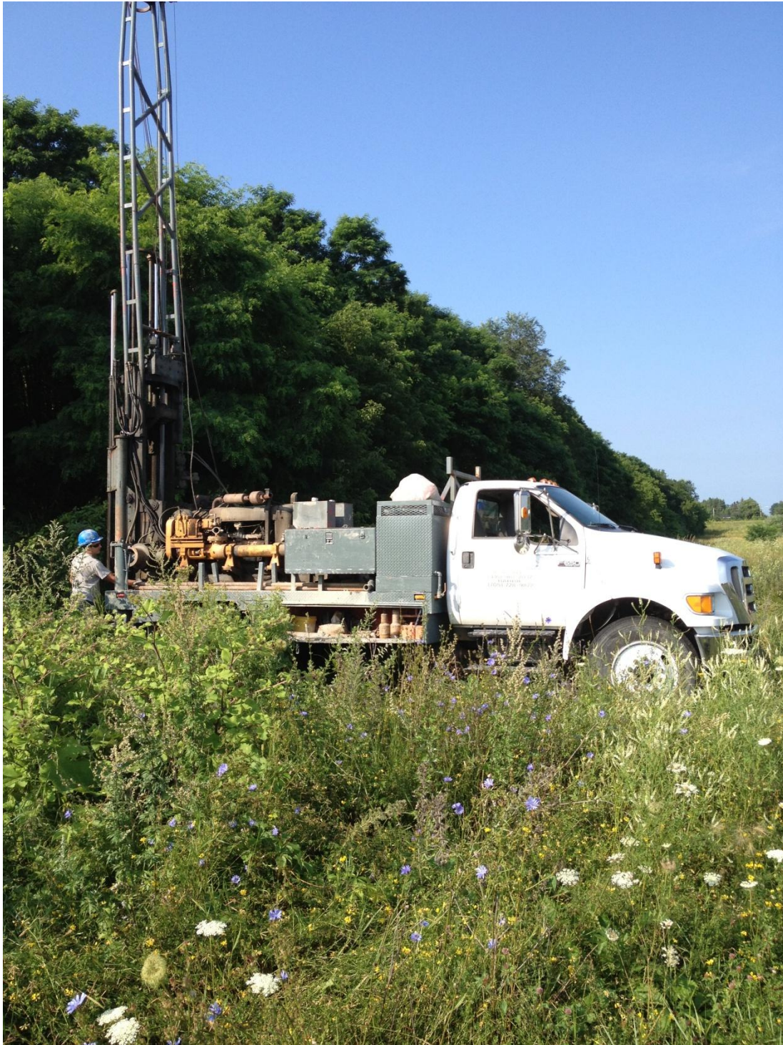
Looking west along bottom of slope and tree line, note incline of slope is parallel with tree tops
