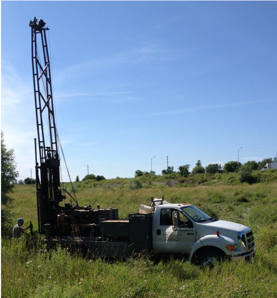
Area of BH 18 representative of central area of Site, note heavy vegetation
