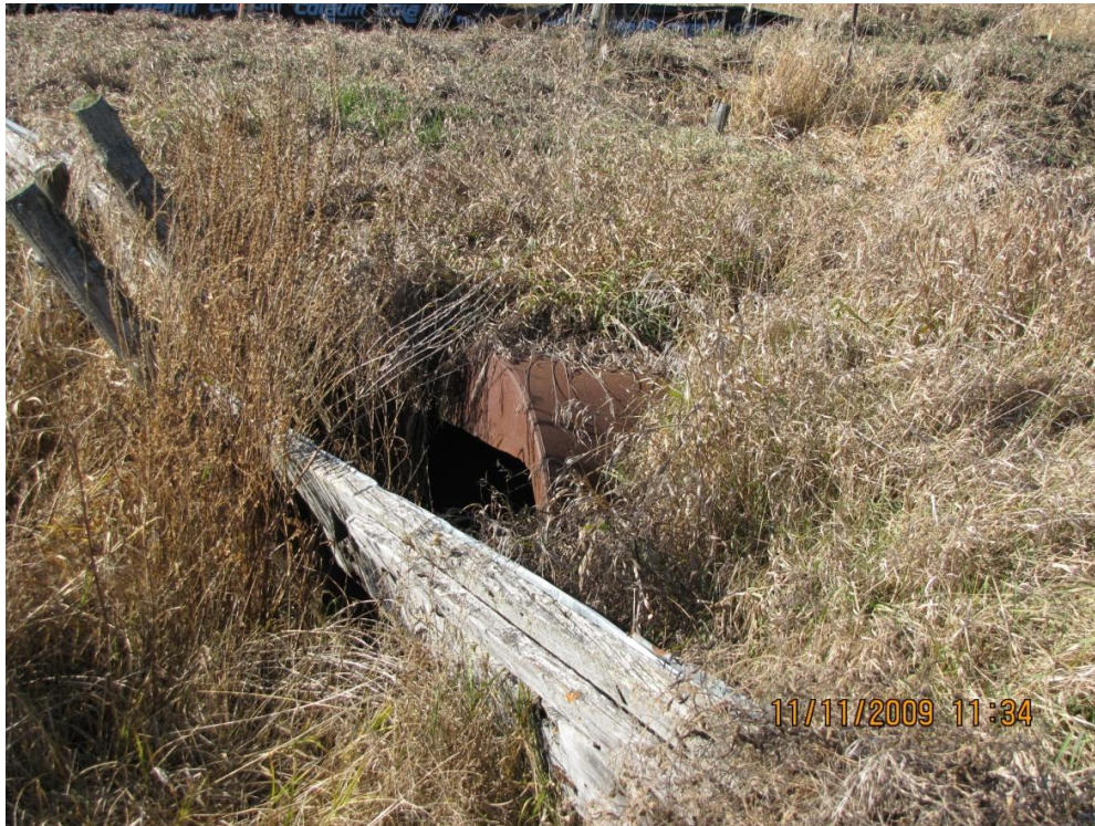
Plate 14: An old boiler or oil tank being re-used as a culvert in the bridge between sections 6D and 6G, looking northwest.
