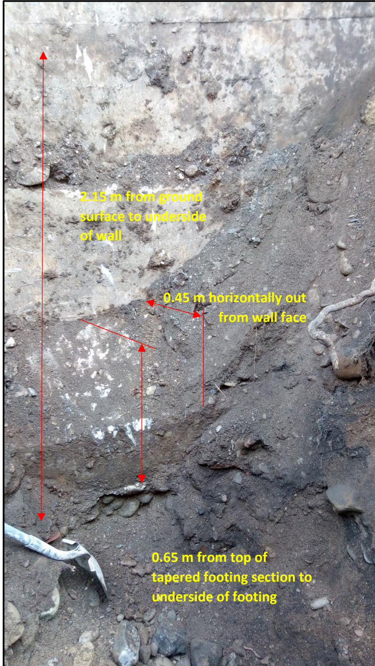
Photo 3 – Details of existing retaining wall abutment system for adjacent section of Somerset Street from field program dated December 2019. Wall abutment placed over engineered granular fill.
