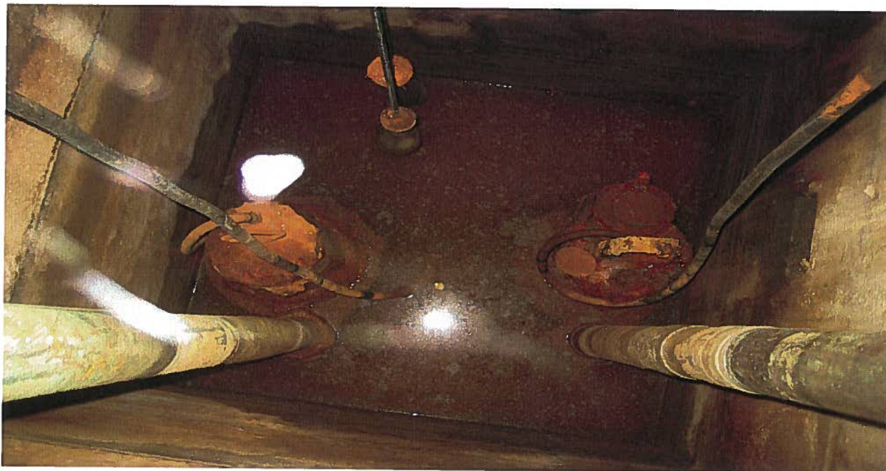
Photograph 9: One of five sumps located in the lowest parking levels. No odours or sheens observed in the sumps.
