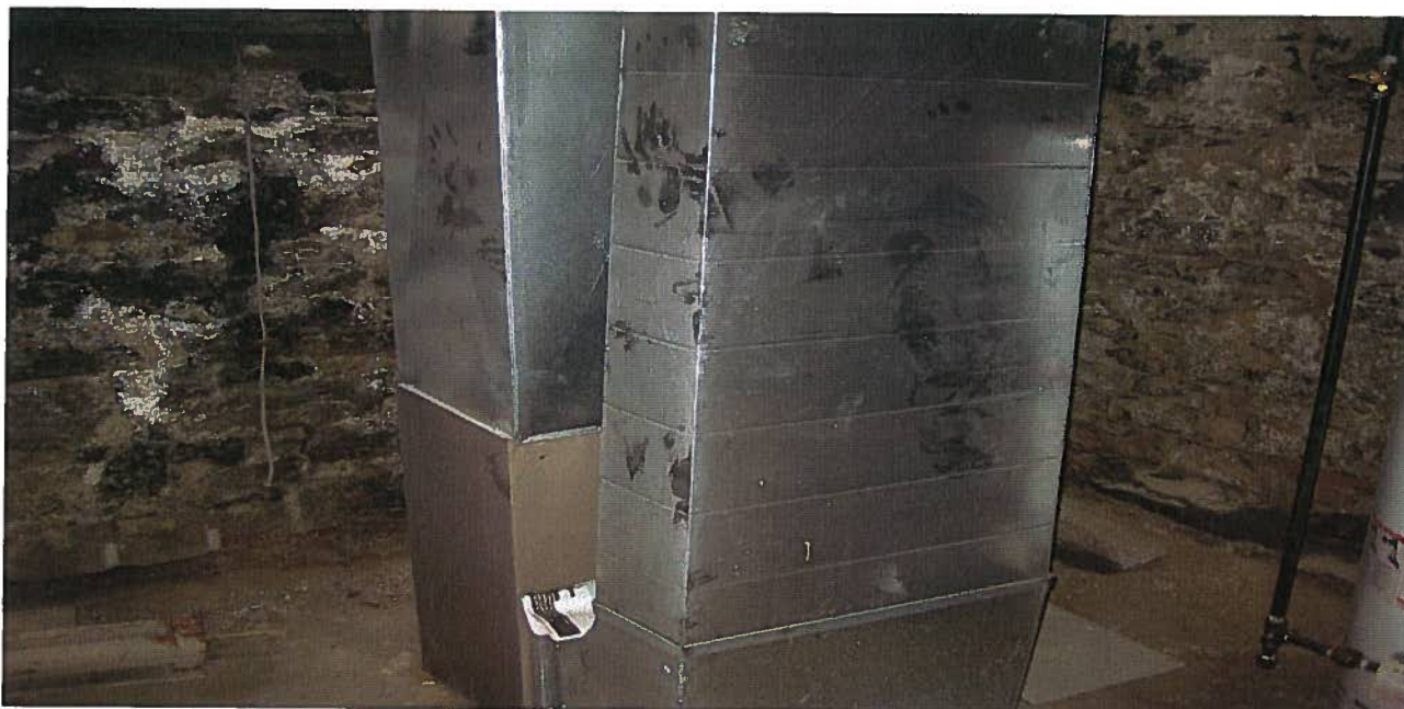
Photograph 15: Furnace located in the basement at 137 Bay Street. The hot water tank is shown to the right.
