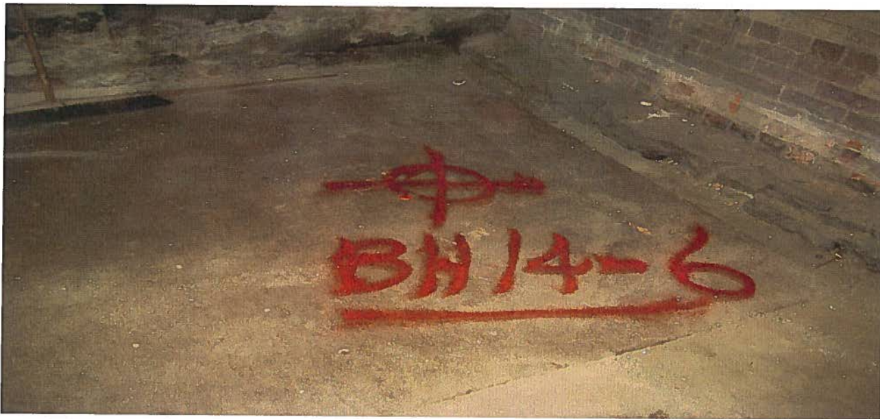
Photograph 17: Mark showing the proposed borehole location for an environmental/geotechnical study in the basement at 137 Bay Street.
