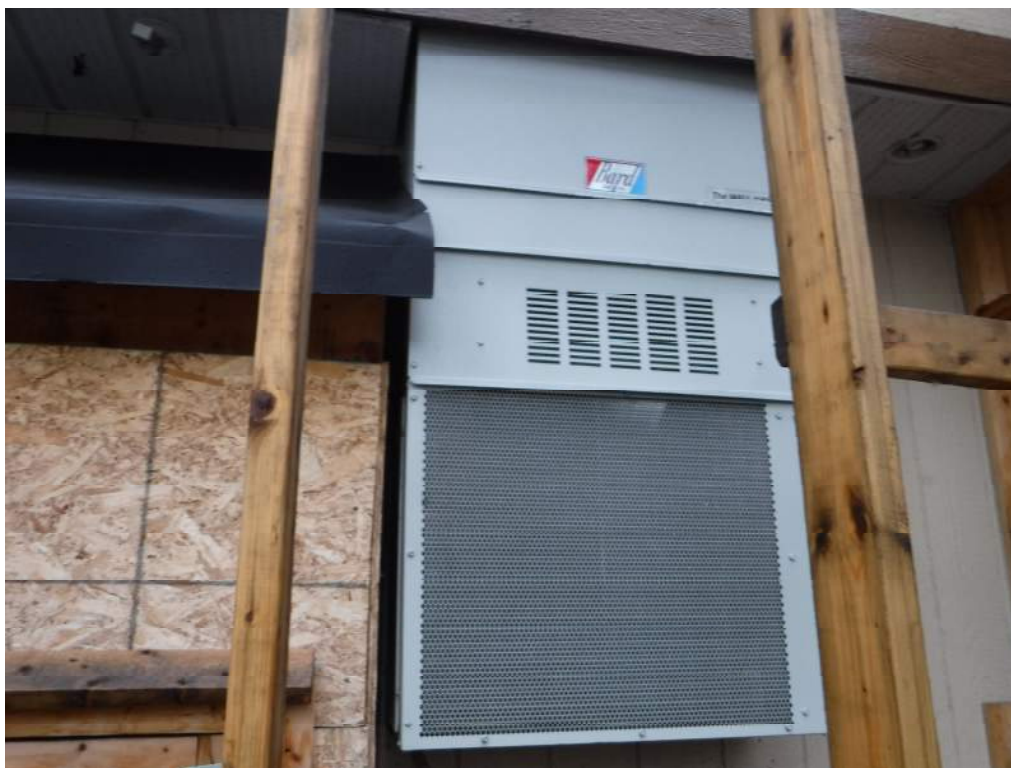
Photograph 7: Air conditioning unit in trailer at Site.
