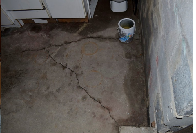
Typical cracked basement slab and water infiltration.
