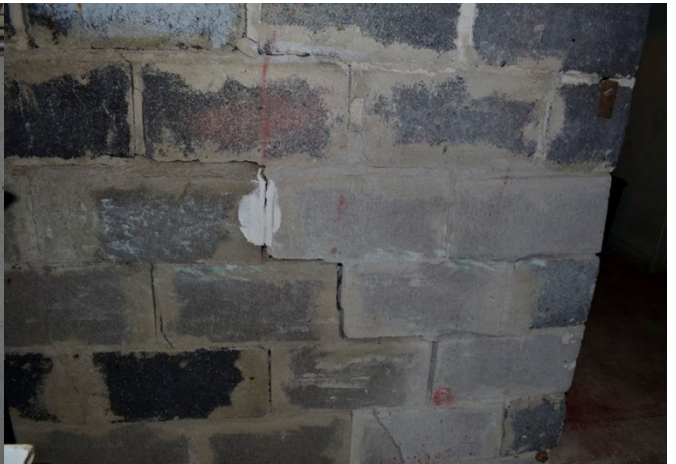
History of crack repairs at basement foundation wall indicates ongoing problem of settlement. Note the concrete block replacements at different periods.
