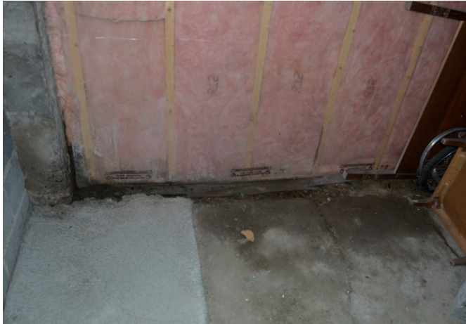
Evidence of repairs and water infiltration at cracked basement slab. Note new slab infill on the left side.
