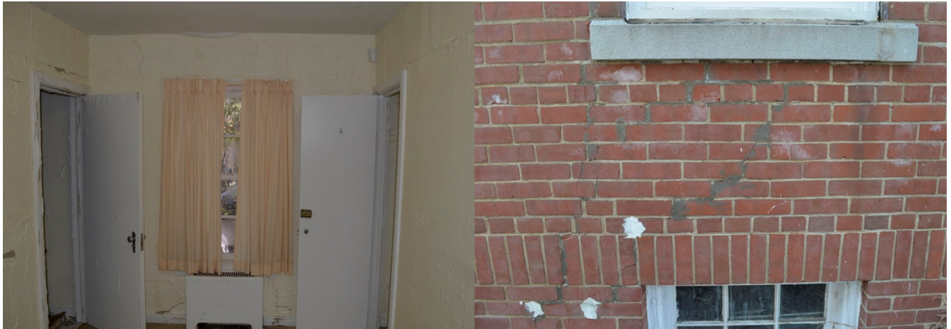
Evidence of water soaked exterior and interior walls. Structural settling and cracking of basement slab, foundation walls and subsequent breach of the building envelope has led to this condition.
