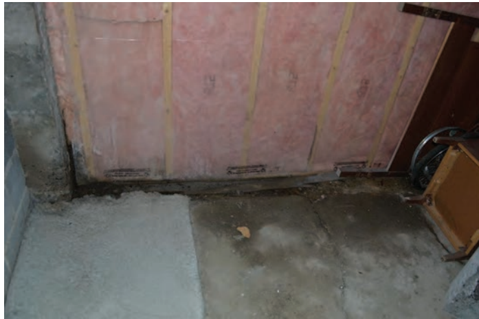
Evidence of repairs and water infiltration at cracked basement slab. Note new slab infill on the left side.
