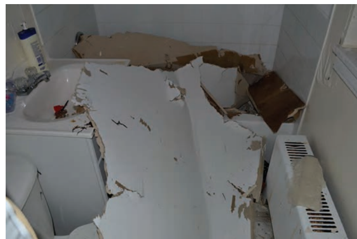
Collapsed drywall ceiling due to water infiltration.
