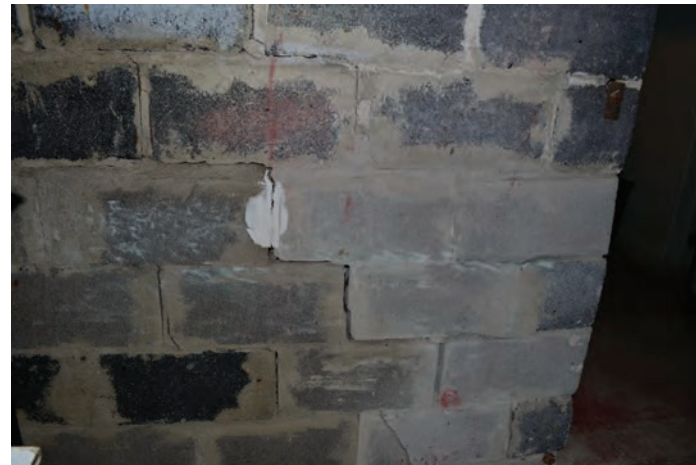
History of crack repairs at basement foundation wall indicates ongoing problem of settlement. Note the concrete block replacements.
