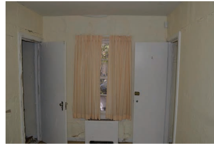
Evidence of water soaked exterior and interior walls. Structural settling and cracking of basement slab, foundation walls and subsequent breach of the building envelope has led to this condition.
