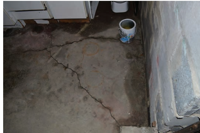
Cracked basement slab and water infiltration.
