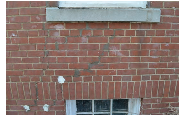
Evidence of extensive cracking and repairs in exterior brick masonry due to failing structure.
