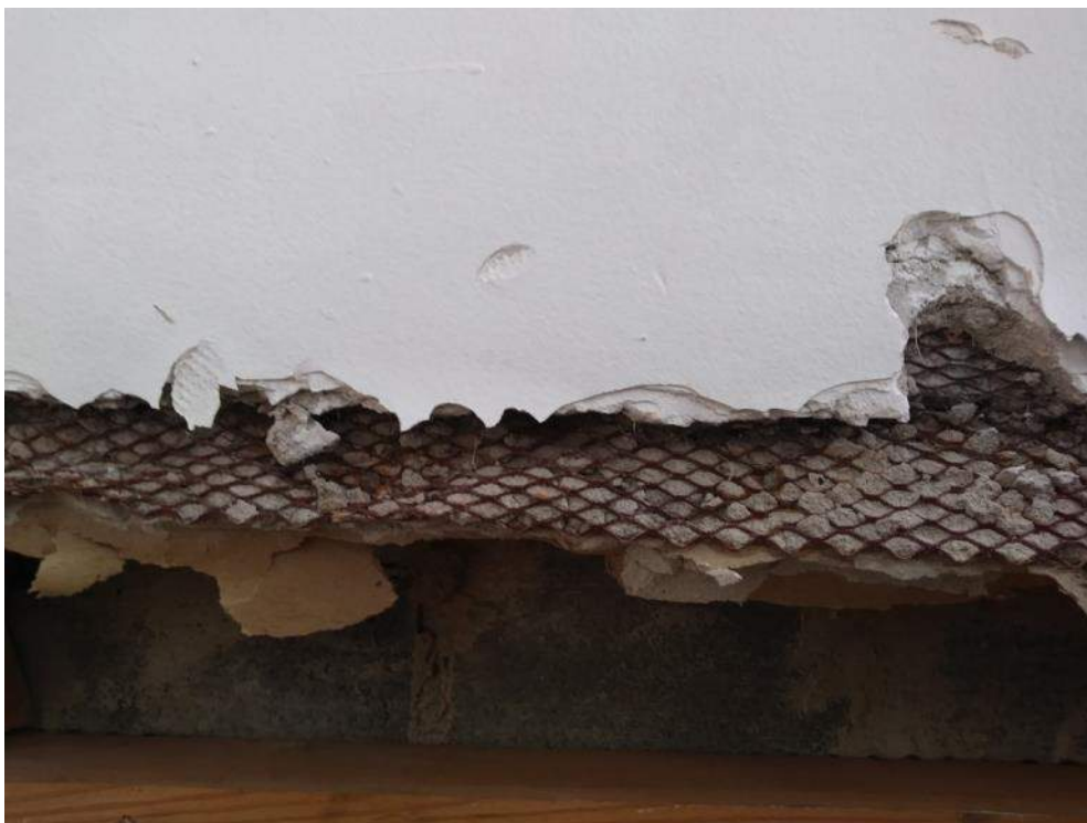
Photo 6: Drywall joints in 208 Prince Albert Street
