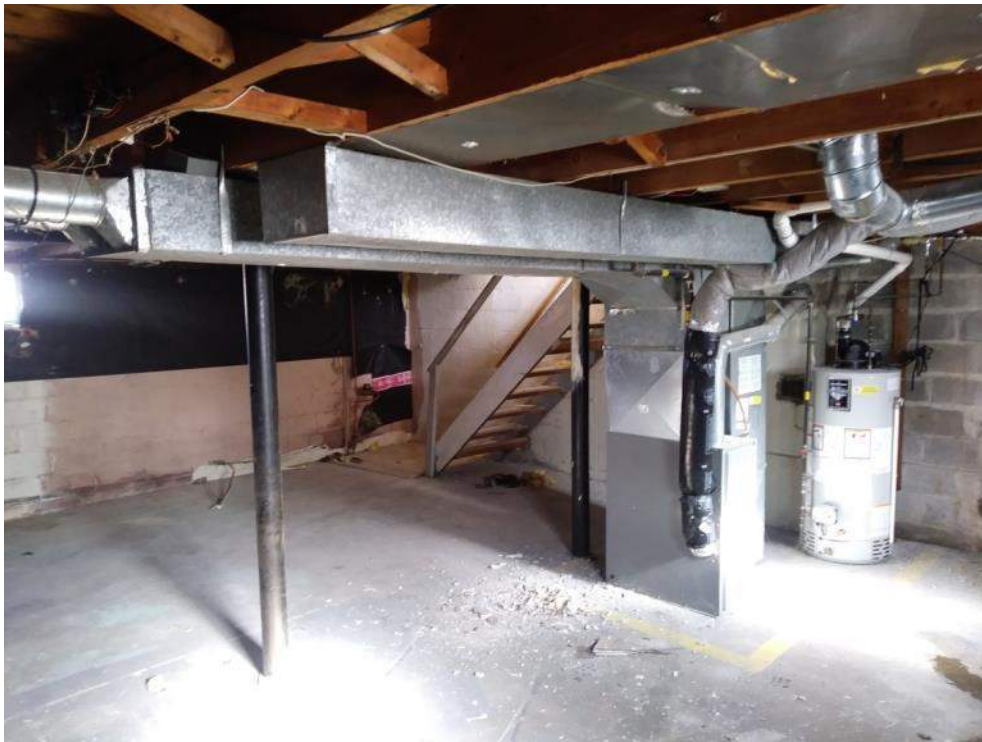
Photo 5: Furnace room in basement of 208 Prince Albert Street (sign on furnace indicates presence of asbestos)
