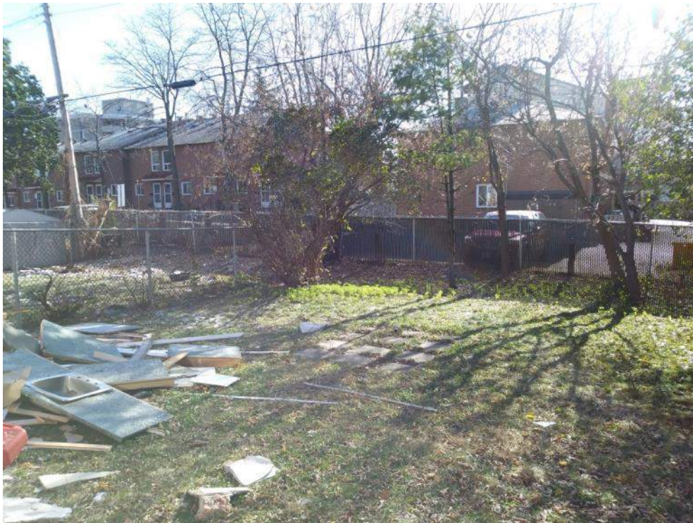
Photo 3: Construction debris in backyard of 208 Prince Albert Street
