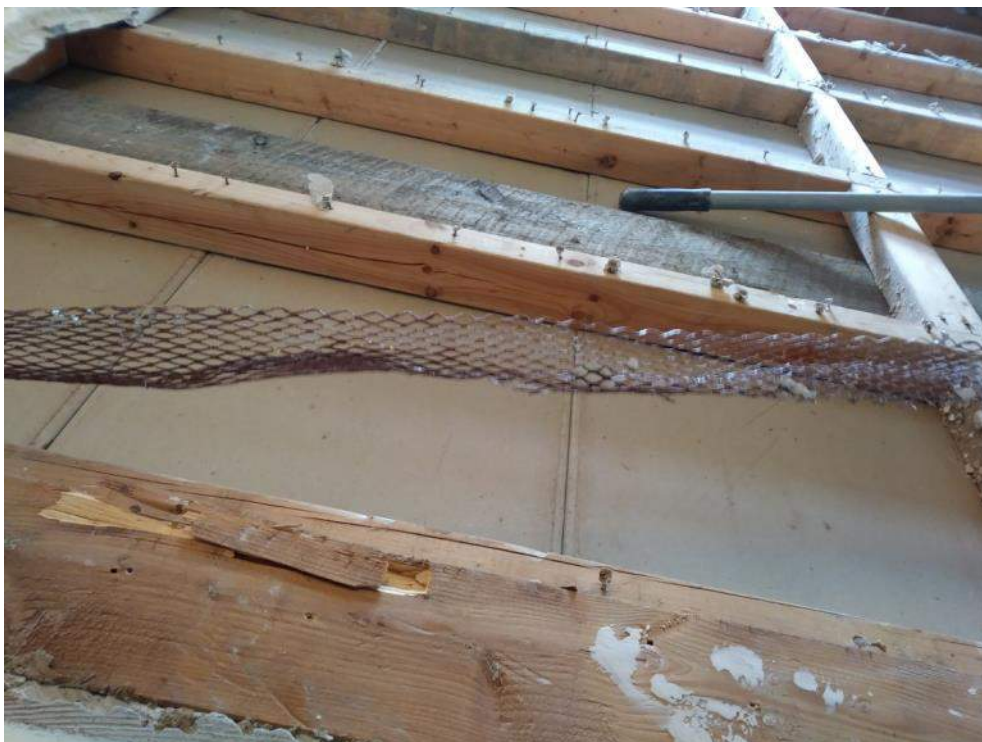
Photo 6: Drywall joints and exposed framing in 210 Prince Albert Street
