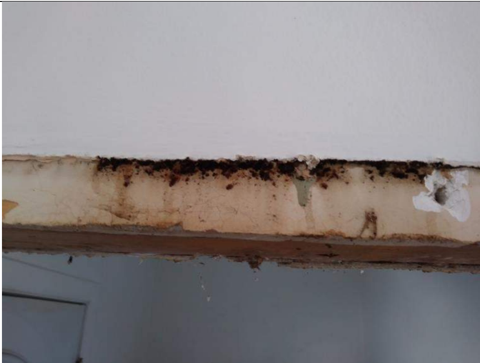
Photo 5: Mould-like substance inside 208 Prince Albert Street, near front entrance
