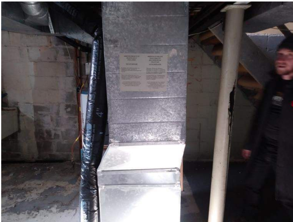
Photo 6: Furnace room in basement of 210 Prince Albert Street (sign on furnace indicates presence of asbestos)
