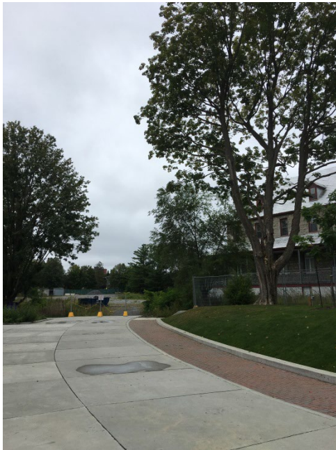
Photo 13: View of new hardscape on north east side of Monastery, looking towards south.
