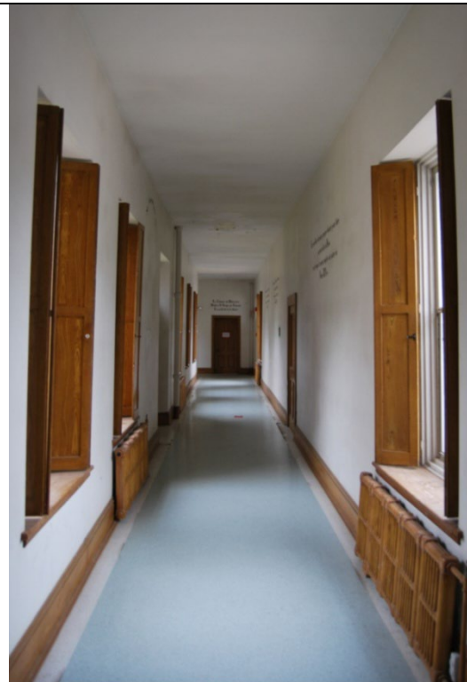
Photo 21: Typical interior corridor of wing (interior partitions to be demolished as part of proposed development).
