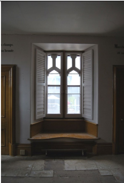
Photo 20: Typical interior view of rectangular window on north wing (windows to be rehabilitated as part of proposed development).
