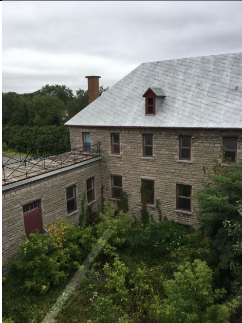
Photo 24: View looking into courtyard from northeast (south wing & southern half of west wing shown here to be removed, courtyard to be infilled in proposed development).
