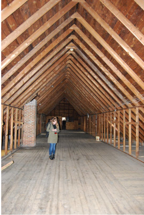
Photo 22: Attic space below hipped roof (to be renovated as office space in proposed development).
