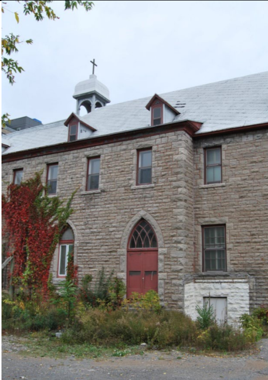
Photo 9: Wall jog in center of on the west wing wall (location of termination of west wing wall in proposed development).
