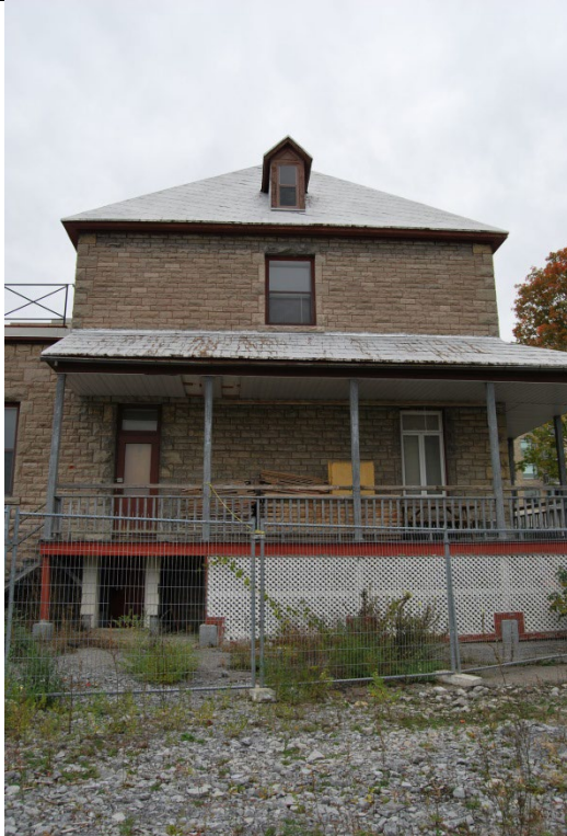
Photo 11: Southern face of east wing from south (to be rehabilitated as part of proposed development).
