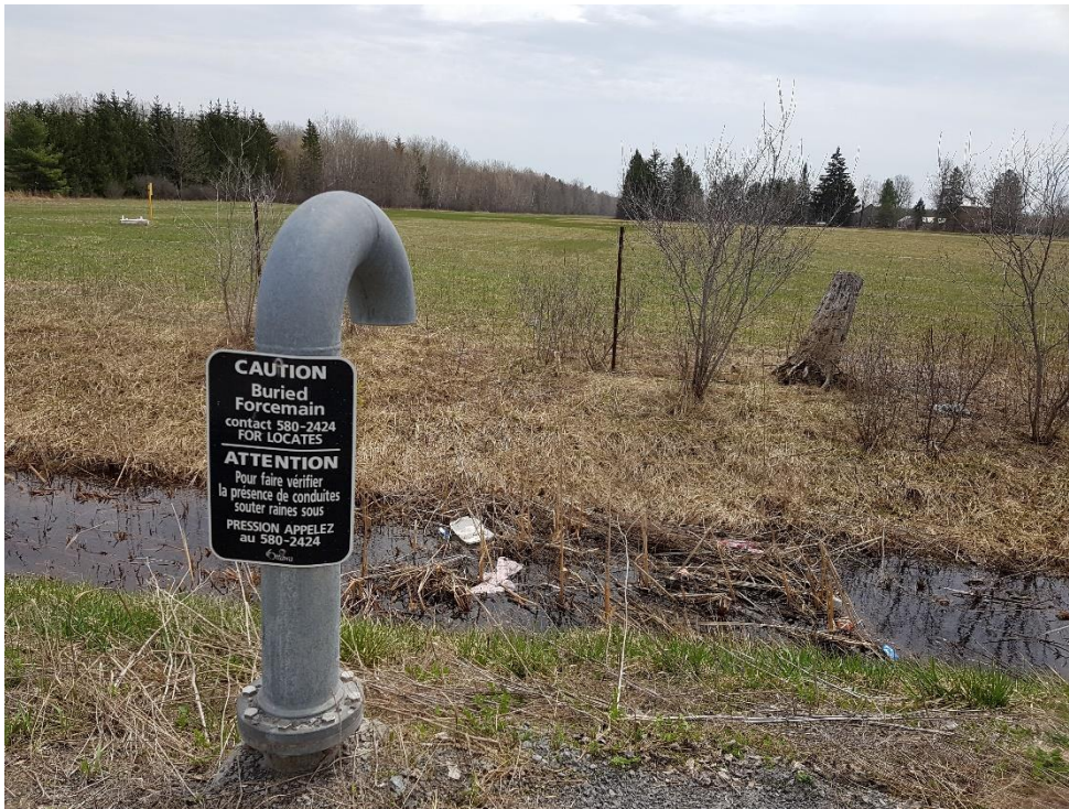
Photo 3: Buried Force-main adjacent to Franktown Road
