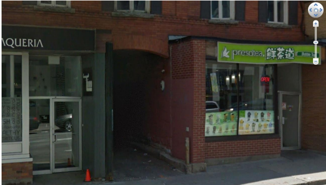
Figure 10: Detail view of the storefront on 208-212 Slater. It would appear that the projecting brick walls, and panel below the storefront window are contemporaneous with a more recent rehabilitation of the storefronts. The same brick detailing is evident on another commercial bay. The original residential configuration consisted of a single window, and door set in the exterior wall aligned with second storey windows. The ground floor exterior walls have been removed, and a beam inserted to support the second floor in order to accommodate the commercial units. The building is classified as a Category 3 heritage resources. Source: Google Earth
