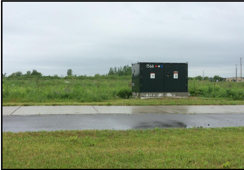
Photograph 5: View of a pad-mounted transformer, located on the south portion of the subject property.
