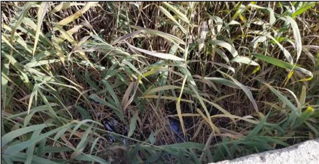
Figure 12: Ditch Below Retaining Wall at North East Side of Property
