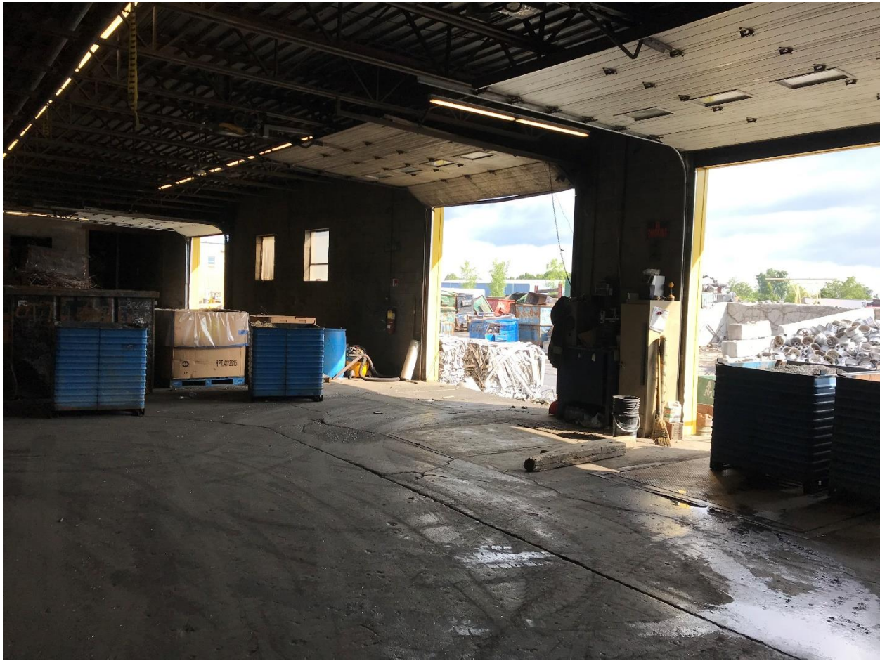
Photograph 2: Looking northeast at the loading docks of the original section of the Main Building (August 2019).
