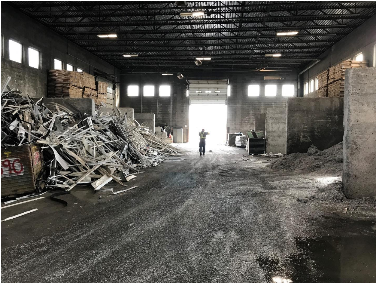
Photograph 6: Looking east at the warehouse storage of metal at the east end of the south branch of the Main Building (August 2019).
