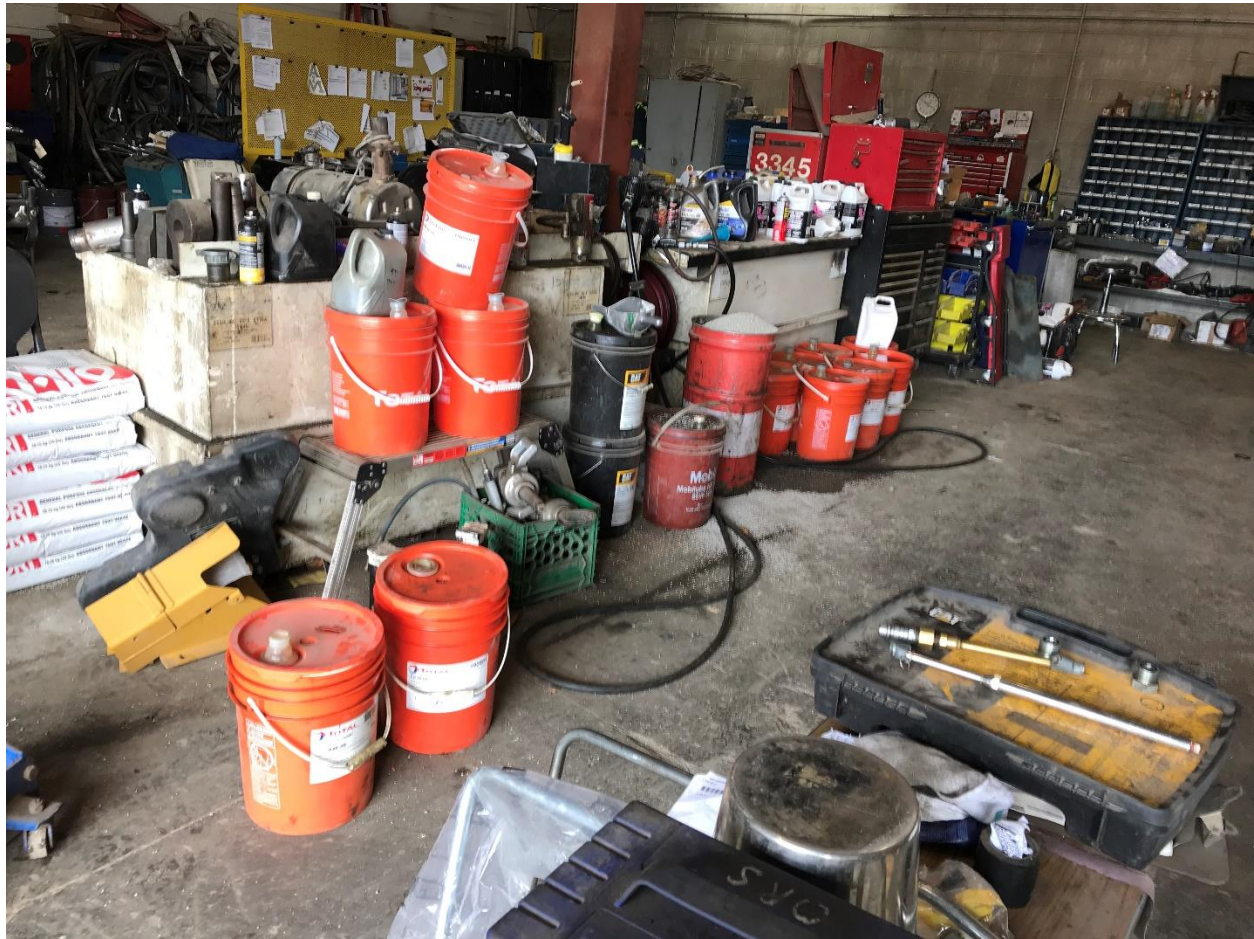
Photograph 22: View inside the garage of the two white ASTs. The one on the left contains hydraulic oil and the one on the right contains engine oil. Pails of hydraulic oil and engine oil around the tanks (August 2019).
