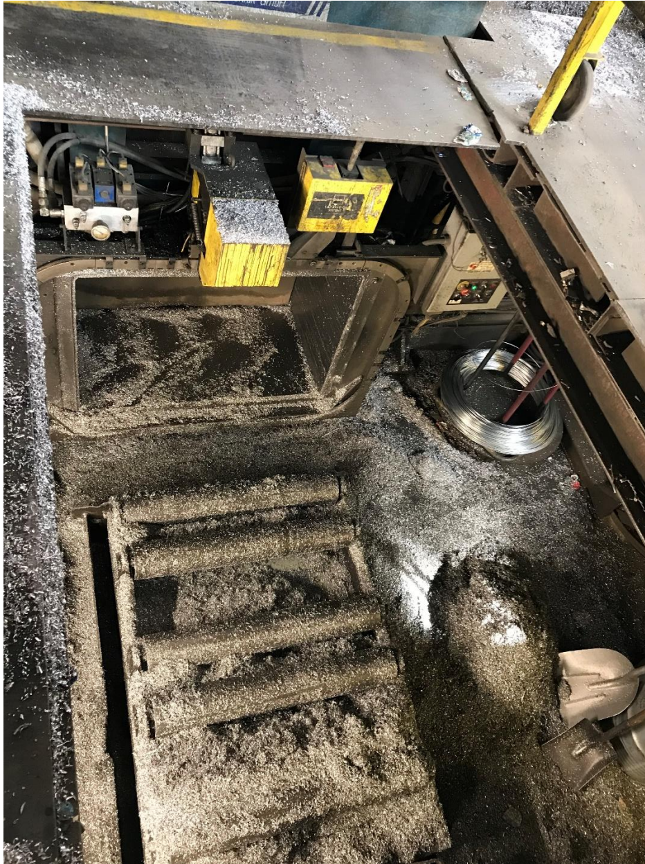
Photograph 5: View of the open hydraulic bailer chamber on the top of the photo, the rollers located on the bottom of the photograph raise up to the warehouse floor for removal of the bailed metal (August 2019)
