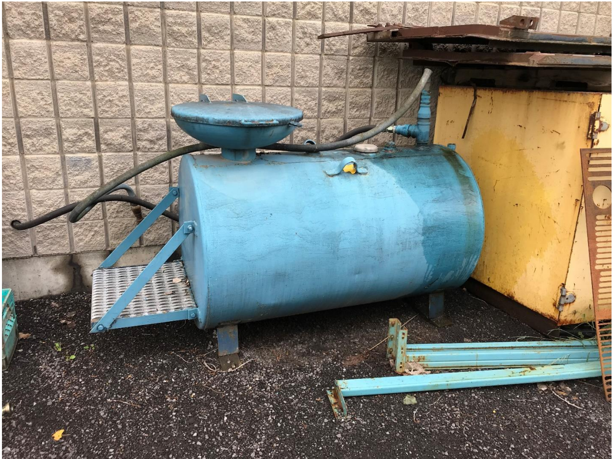
Photograph 23: Waste oil AST on the north side of the Garage Building. There was water on the right side of the tank from the rain water dripping from the sheet metal (August 2019).
