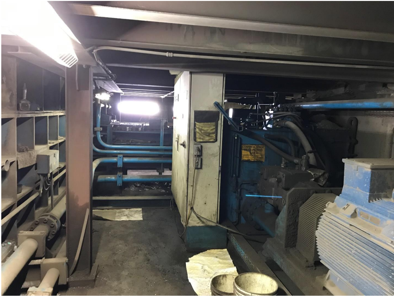
Photograph 8: Looking west at the hydraulic oil AST (blue tank on the right hand side) connected to the hydraulic bailer at the southwest corner of the Main Building (August 2019).
