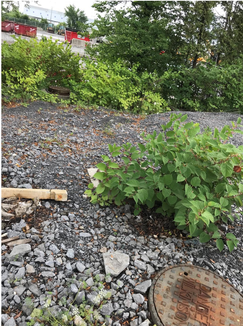
Photograph 13: Looking south at the location of the oil/water separator and discharge to the storm sewer that runs along the south property line (August 2019).
