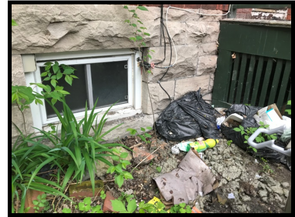
Photo 6: The Phase One Property (24 Pretoria Avenue – domestic waste within front yard)
