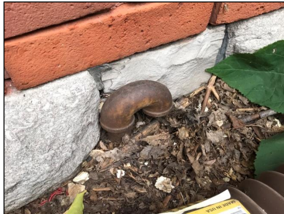
Photo 5: The Phase One Property (28 Pretoria Avenue – historical heating oil AST fill/vent pipe, exterior west wall)
