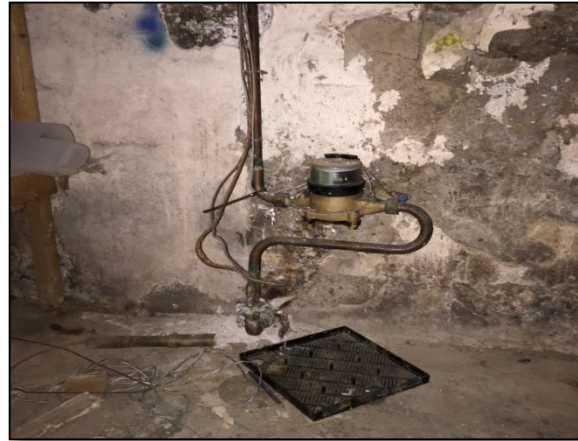
Photo 14: The Phase One Property (30 Pretoria Avenue – general interior view of basement remaining heating oil AST connections)
