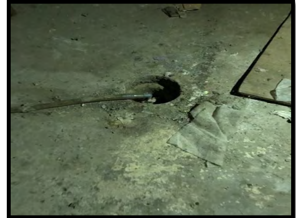
Photo 3: The Phase One Property (24 Pretoria Avenue – basement floor drain)
