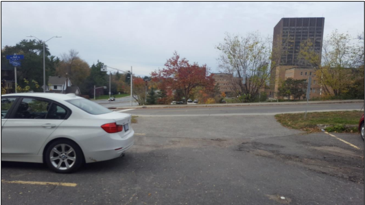
Photograph 14: Photo of damaged asphalt near parking lot entrance (October 27, 2016).
