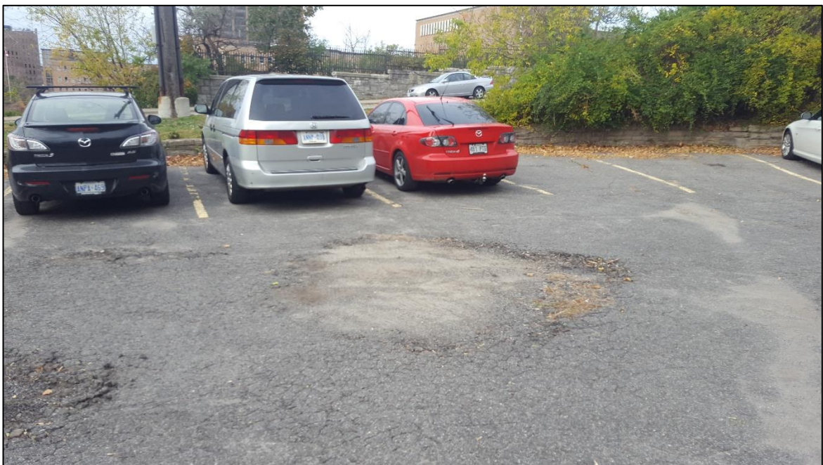
Photograph 13: Photo of worn and damaged asphalt (October 27, 2016).
