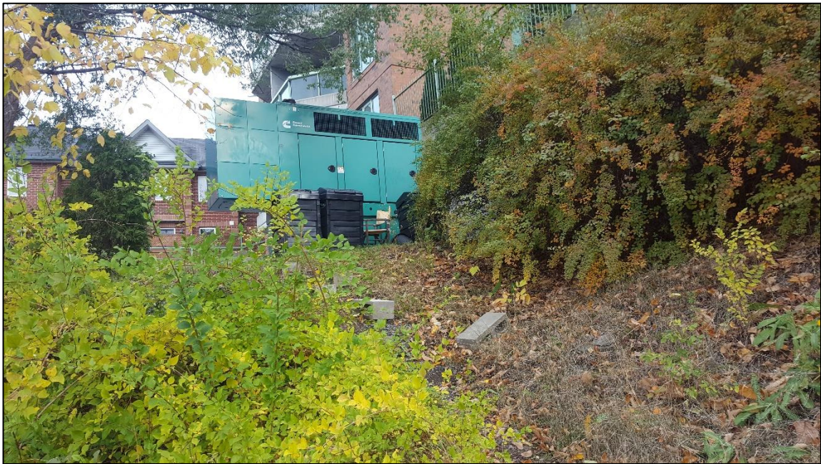
Photograph 12: View of diesel generator locate on east adjacent property (October 27, 2016).
