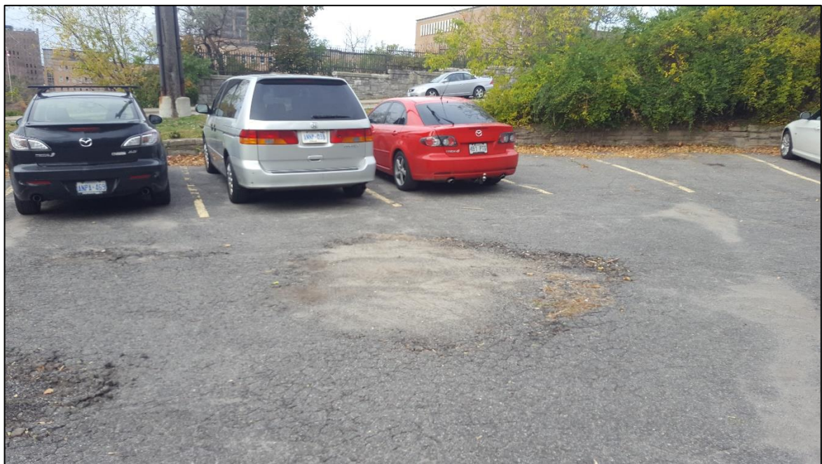
Photograph 13: Photo of worn and damaged asphalt (October 27, 2016).
