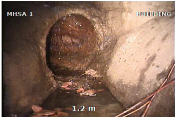
Figure 4 – 300mm diameter storm service
