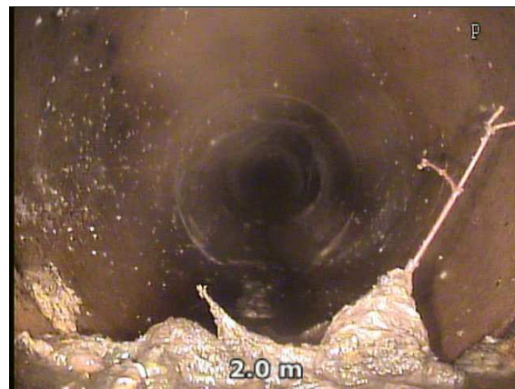
Figure 7 – Partial blockage (2.0m from MHSA1)
