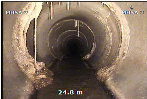
Figure 14 – Encrustation at pipe joints
