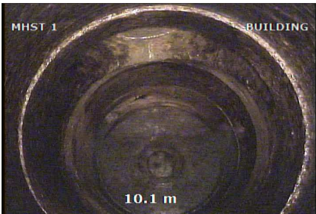
Figure 18 – Cast-iron service from building
