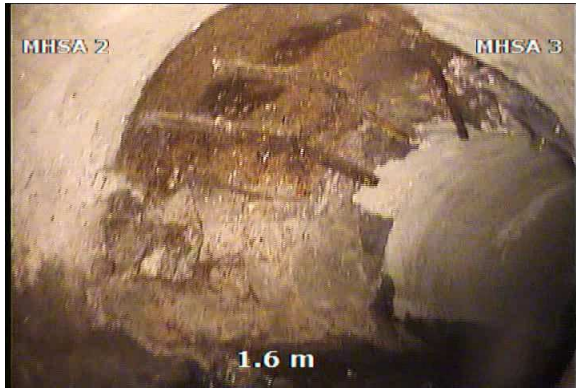
Figure 12 – Rebar exposed at MH-pipe joint
