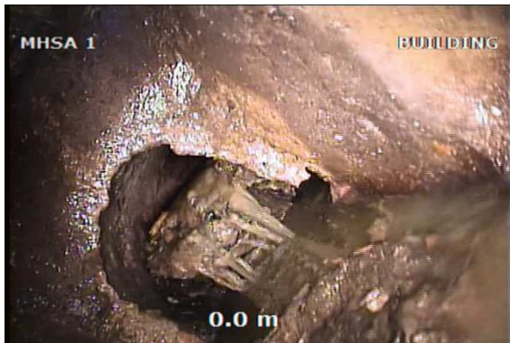
Figure 2 – Misaligned with MHSA1 invert
