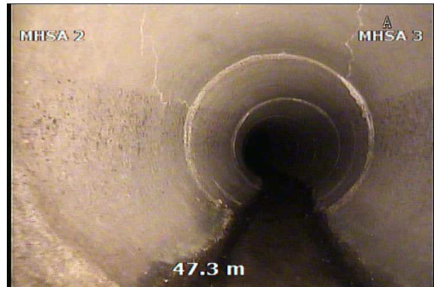
Figure 15 – Minor cracking at 9 and 1 o'clock
