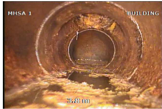
Figure 5 – Sanitary backflow in abandoned storm service
