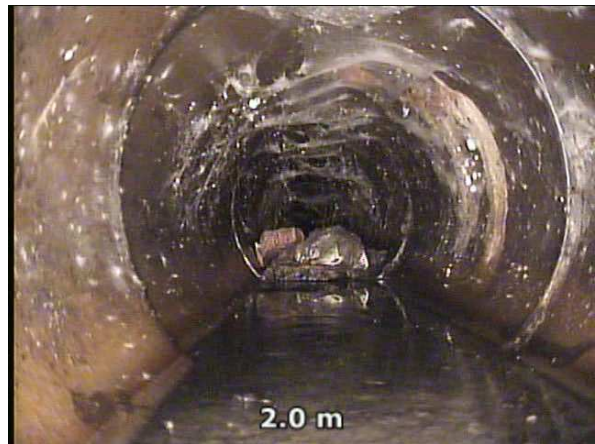
Figure 11 – Partial blockage approximately 6m from MHS A2
