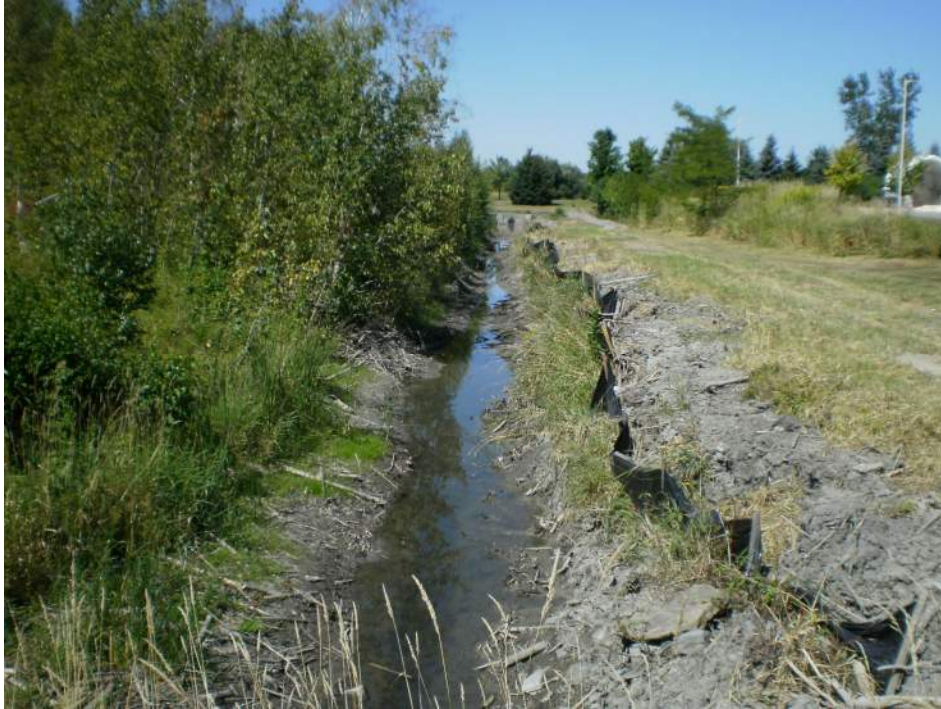
Photo 7 – North-south stormwater channel in the stormwater easement in the east edge of the site. View looking north from Solandt Road
