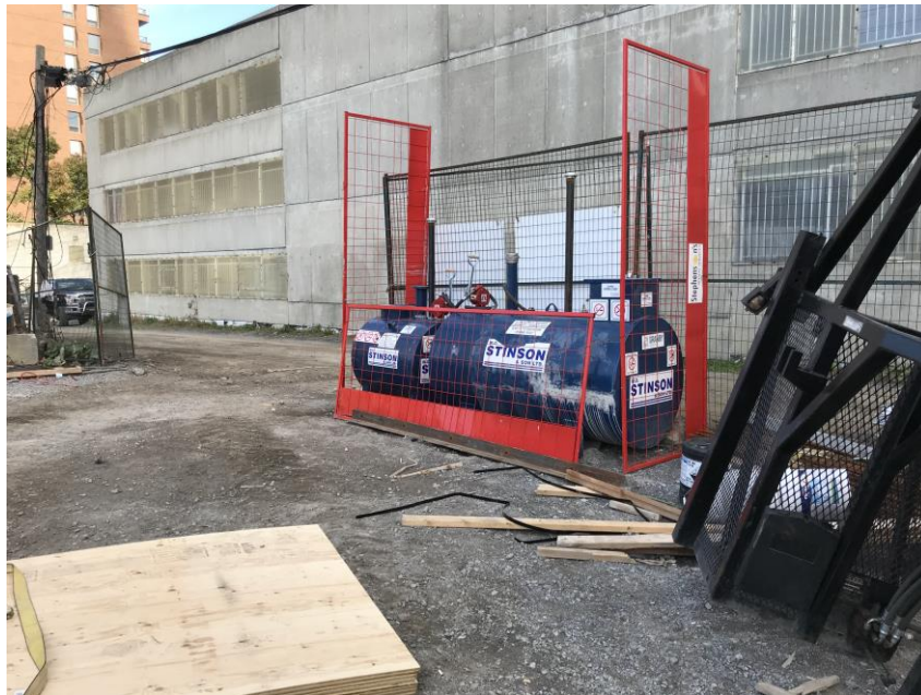
Photo 3: Temporary AST containing gasoline and diesel, located along the eastern property boundary.
