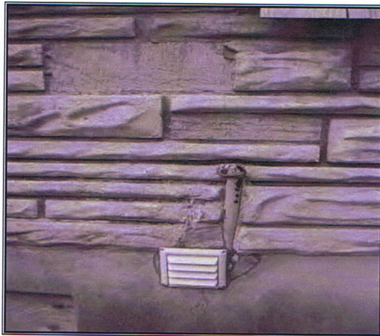
Photo 5 – Fill/vent pipe embedded in the exterior concrete wall at the southeast corner of Site Building B.
