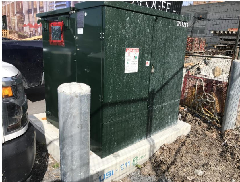
Photo 2: Electrical transformer along the western side of the Property.
