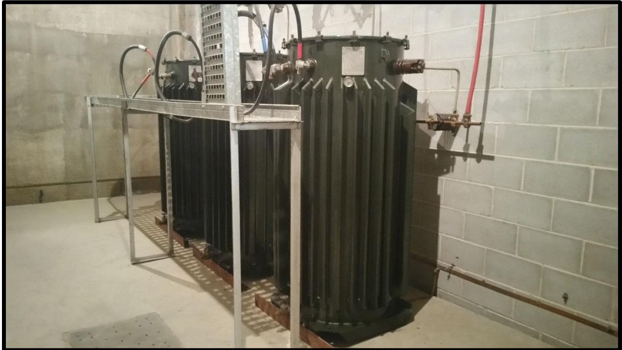
Photograph 5: Photograph of interior transformers in the electrical room on the lower level of the Rideau Carleton Raceway building.
