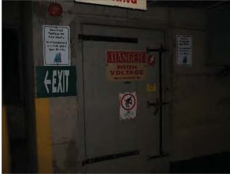
Photo 3 – Transformer vault located on the first basement level of the Site Building (PCA/APEC).
