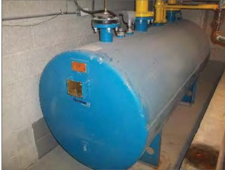
Photo 1 – 1,250-L diesel AST located within the emergency generator room in the second basement level (PCA/APEC).
