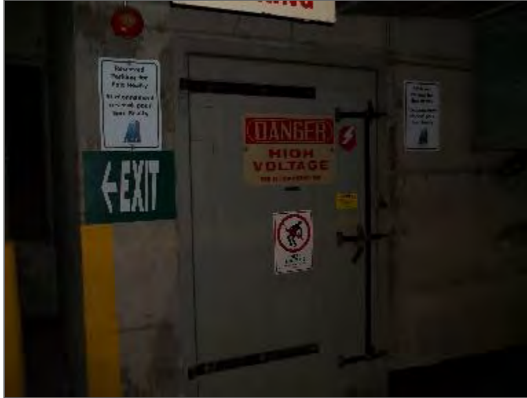
Photo 3 – Transformer vault located on the first basement level of the Site Building (PCA/APEC).
