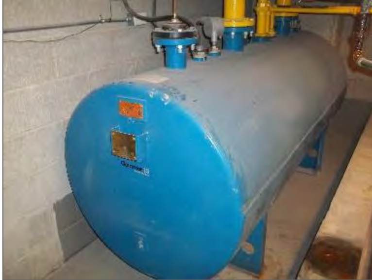
Photo 1 – 1,250-L diesel AST located within the emergency generator room in the second basement level (PCA/APEC).
