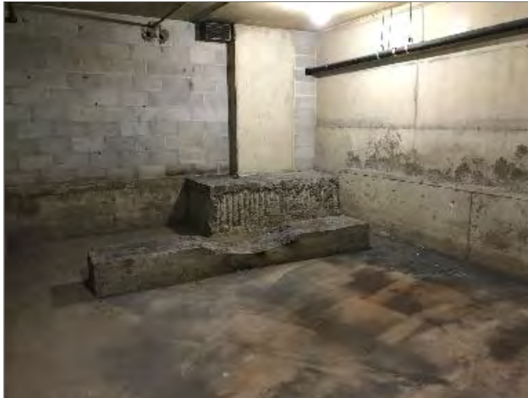
Photo 2 – Formerly-used 'tank room' within the second basement level, where a former heating oil AST was located (PCA/APEC).
