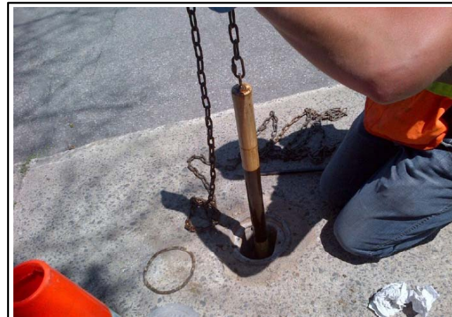
Photo 8 - Passive Hydrophobic Petro-Bailer at BH12
