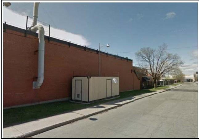
Photo 1 - DPE System Treatment Shed
