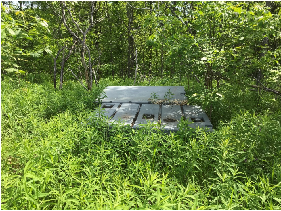
Photo 9 – View of two plastic tanks on east side of Property; view is facing east.
