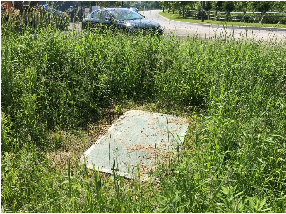
Photo 3 – View of Bell access hatch on southwest portion of Site; view is facing south.
