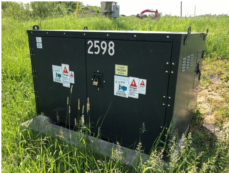
Photo 6 – View of generator in northwest corner of Property; view is facing southeast.
