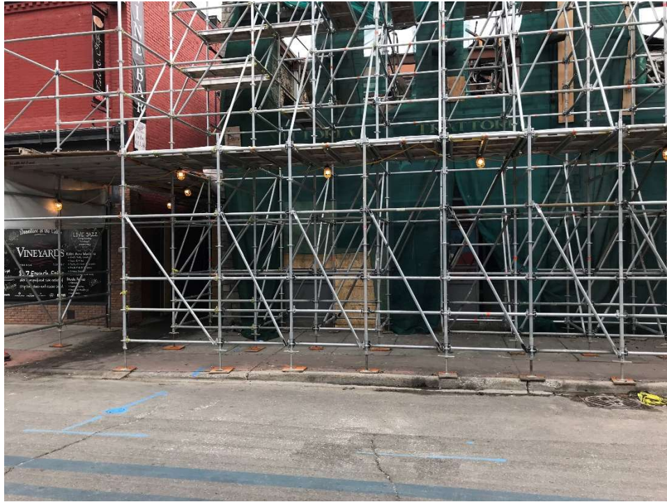
Photograph 1: View of west face of 35-37 William Street, facing northeast. Photo illustrates scaffolding placed during rehabilitation works subsequent to the April 2019 fire and adjacent commercial property to the north.
