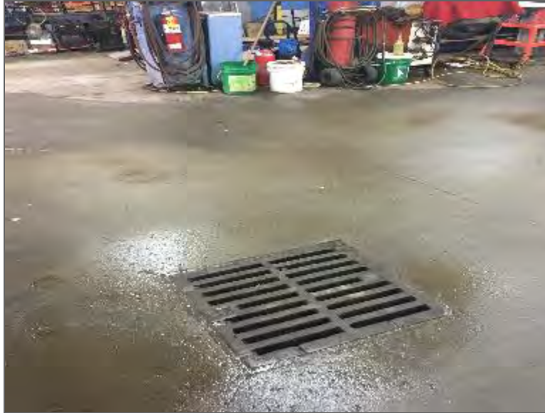
Photo 15 – Single-stage oil/water separator located within the operating automotive repair/servicing operation (i.e., Gifford's Automotive).
