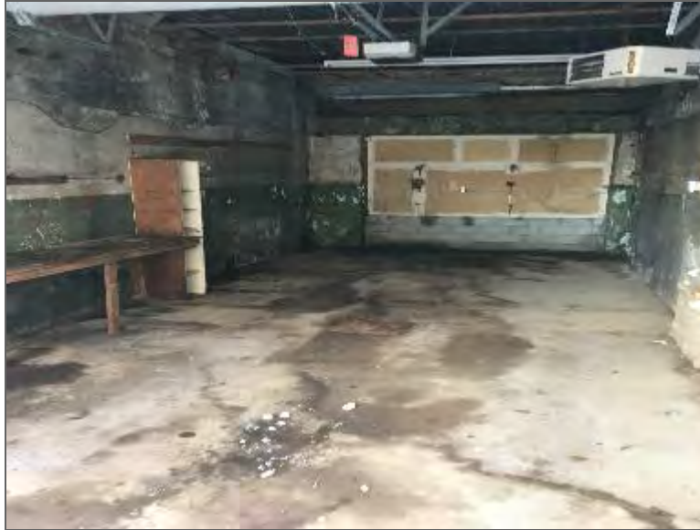
Photo 11 – Former spray painting area within the north-northwest portion of Site Building A.
