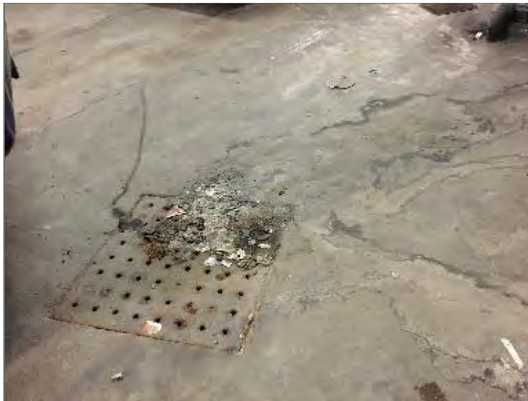
Photo 8 – Single-stage oil/water separator located within the former automotive repair/servicing facility (i.e., Auto Re-Bex).
