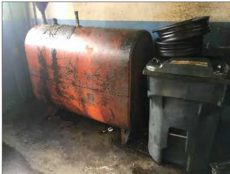
Photo 14 – A 910-L waste oil AST located along the south wall of the tenant space occupied by Gifford's Automotive.
