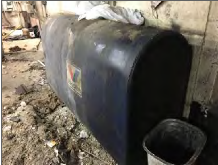
Photo 9 – A 910-L waste oil AST located along the south wall of the tenant space formerly occupied by Auto Re-Bex.
