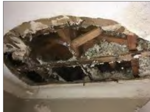
Mould present on the back side of the drywall/textured plaster ceiling finish in the front entrance at 315 Tweedsmuir Avenue.
