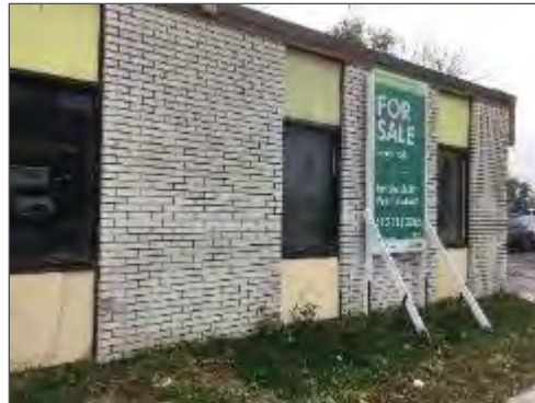
Asbestos-containing cement board present above and below the windows along Office 1 & 2 at 320 McRae Avenue.
