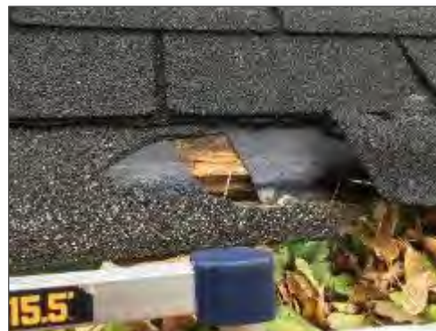
Non-asbestos tar paper present in the roof at 315 Tweedsmuir Avenue.
