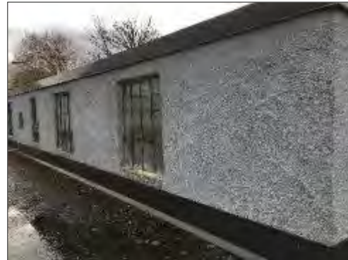
Asbestos-containing aggregate-embedded stucco present on the exterior walls of Storage 2 on the roof level at 320 McRae Avenue.
