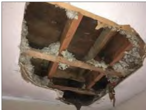
Mould present on the back side of the drywall/textured plaster ceiling finish in the front entrance at 315 Tweedsmuir Avenue.
