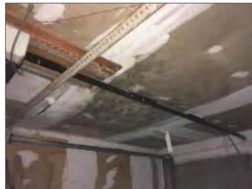
Mould present on the drywall ceiling in the separate Garage at 315 Tweedsmuir Avenue.
