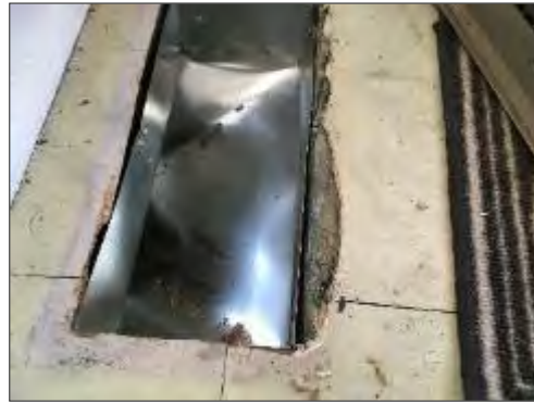
Asbestos-containing vinyl sheet flooring present as the base layer in the front entrance at 311 Tweedsmuir Avenue.
