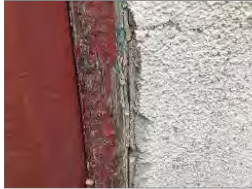
Asbestos-containing white caulking present around the south exterior door frame frames at 320 McRae Avenue.
