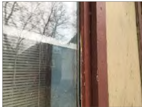
Asbestos-containing blue caulking present around the exterior window frame on the Garage at 315 Tweedsmuir Avenue.
