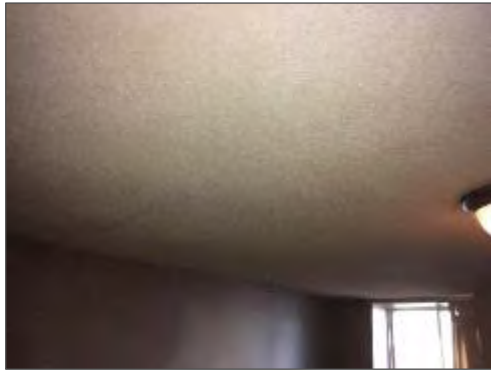
Non-asbestos ceiling stipple present throughout the basement at 315 Tweedsmuir Avenue.
