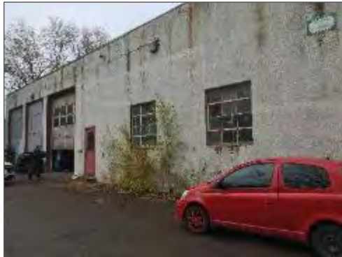
Asbestos-containing aggregate-embedded stucco present on the exterior walls of Garage 2 and Storage 2 at 320 McRae Avenue.
