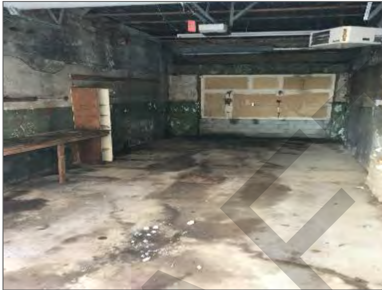
Photo 11 – Former spray painting area within the north-northwest portion of Site Building A.
