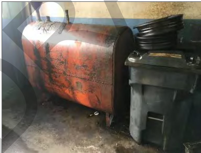
Photo 14 – A 910-L waste oil AST located along the south wall of the tenant space occupied by Gifford's Automotive.
