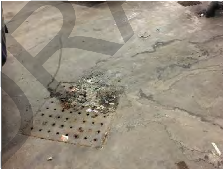
Photo 8 – Single-stage oil/water separator located within the former automotive repair/servicing facility (i.e., Auto Re-Bex).
