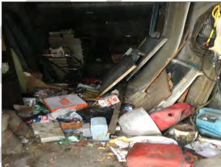
Photo 10 – Former flammable liquid storage area within the northwest portion of Site Building A.
