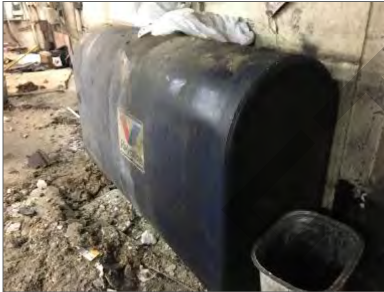
Photo 9 – A 910-L waste oil AST located along the south wall of the tenant space formerly occupied by Auto Re-Bex.
