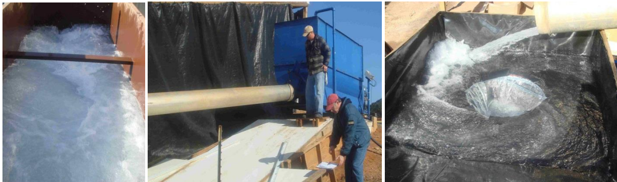
Inside View of Hopper Agitator
