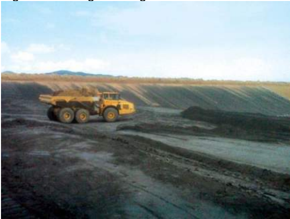
Figure 17. Large un-vegetated surfaces
