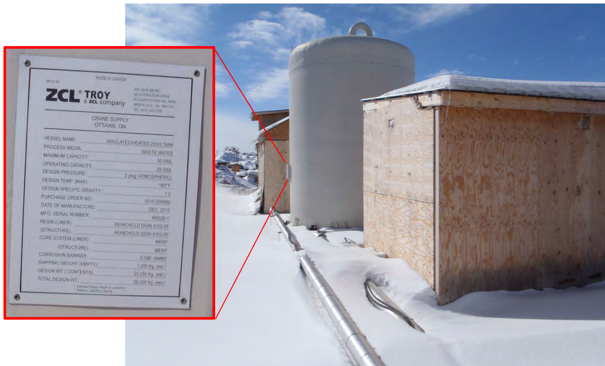
Photograph 7: Insulated/Heated Waste Water holding tank for the water treatment system.
