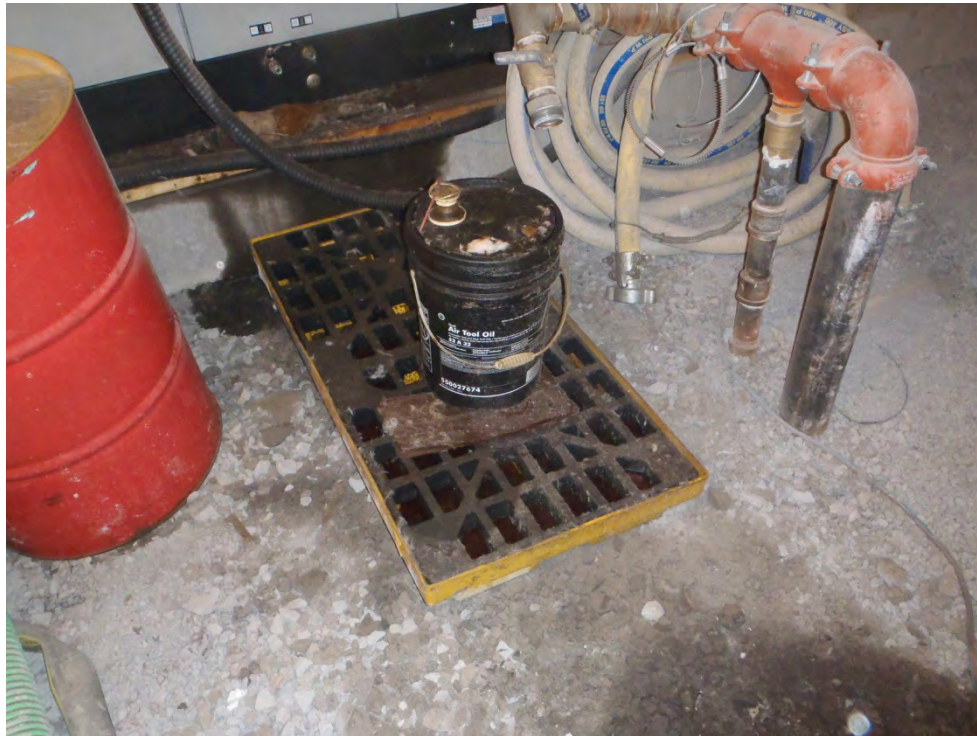
Photograph 5: 20 L pail of Air Tool Oil with secondary containment inside water treatment system building. Note staining on concrete and on gravel surface.
