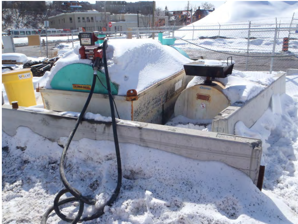
Photograph 19: 455 L diesel AST and 136 L waste oil AST located west of the shop/garage. Two documented spills have occurred in this area.
