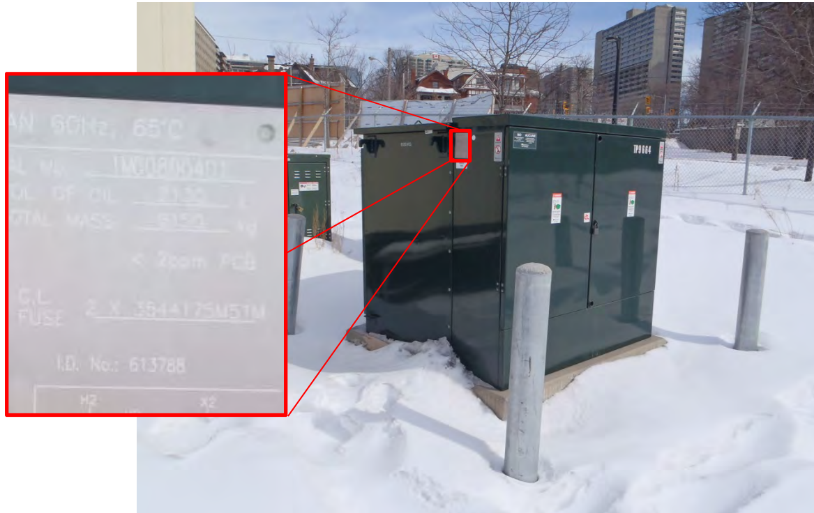
Photograph 31: Transformer containing “<2 ppm PCB” located near the northeast corner of the Site.
