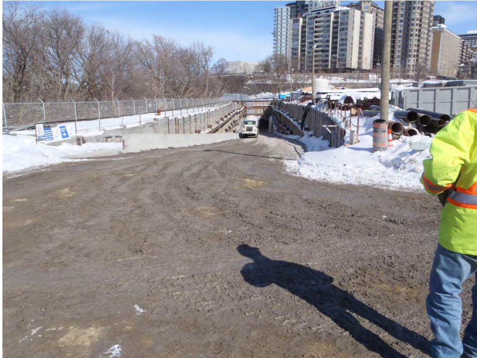
Photograph 17: 'West Portal' tunnel operations for the OLRT, adjacent to the north of the Site
