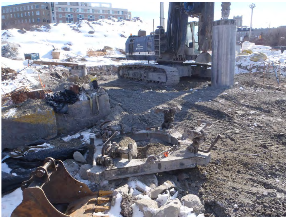
Photograph 14: CSST shaft construction on the southeast corner of Wellington Street and the OC Transpo Transitway with fill pile in background.
