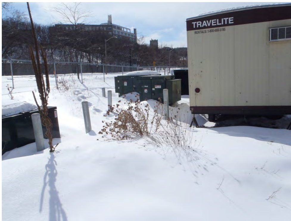
Photograph 2: Transformer boxes located behind a site trailer in the northeast corner of the Site.
