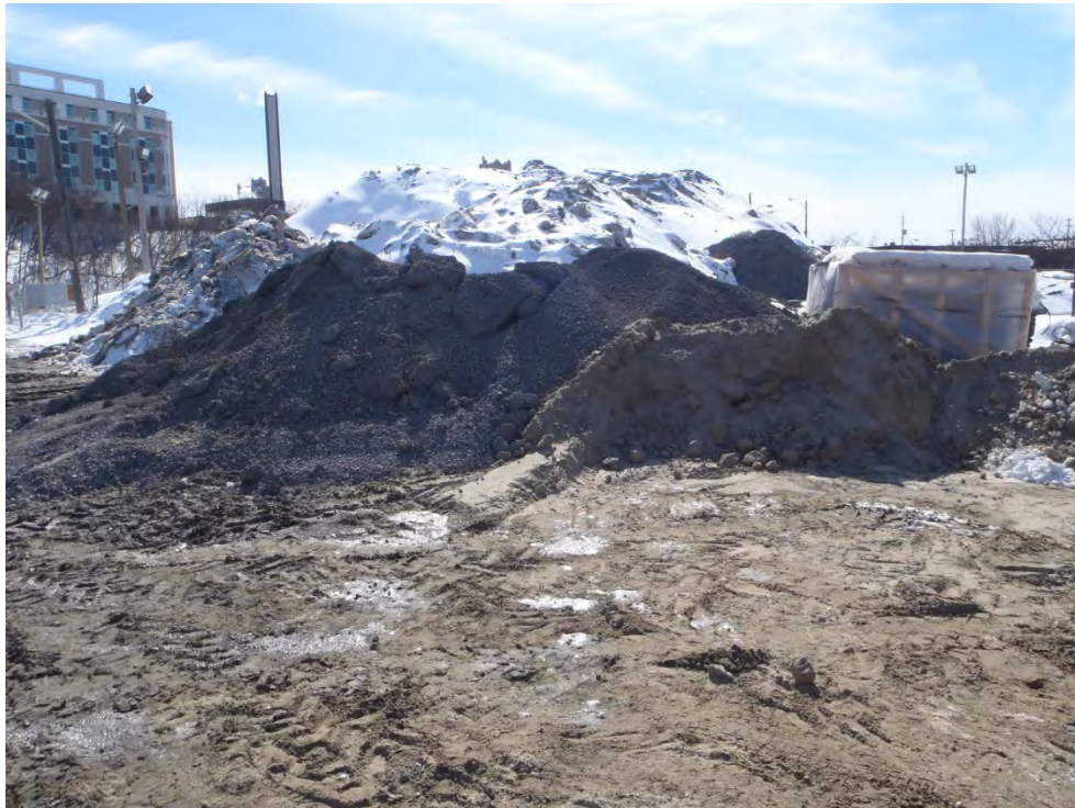
Photograph 13: Fill pile located on the part of the Site between Brickhill Street and the OC Transpo Transitway
