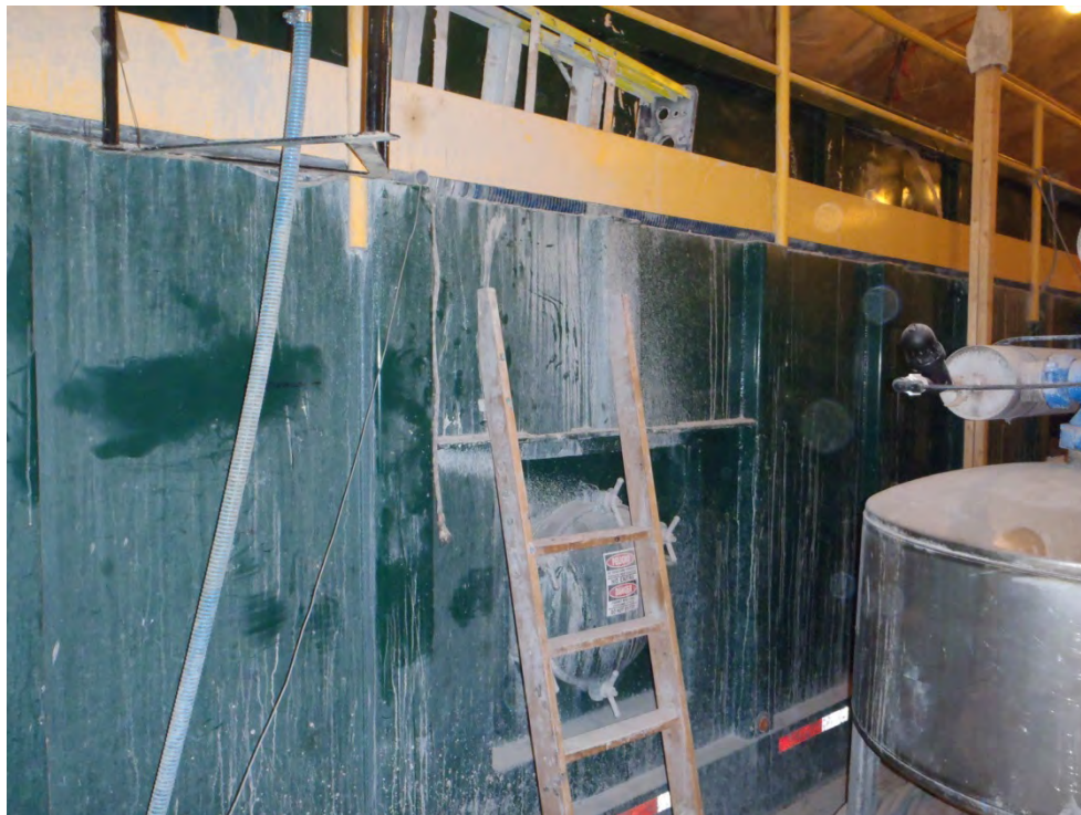
Photograph 6: Water filter/clarifier treatment system.
