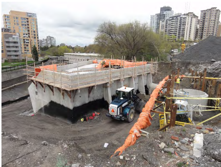
Photo 10 – View of tunnel construction work associated with the CSST, located immediately southwest of the Site.
