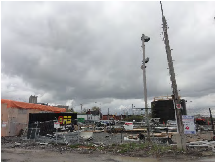
Photo 14 – View of CSST construction area located adjacent south of the Site, looking southwest.
