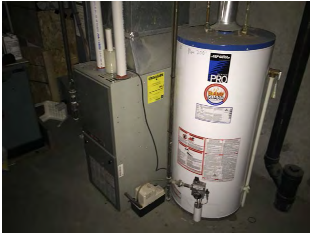
Example of natural gas powered furnace and water heater at 14 Dunbar Court
