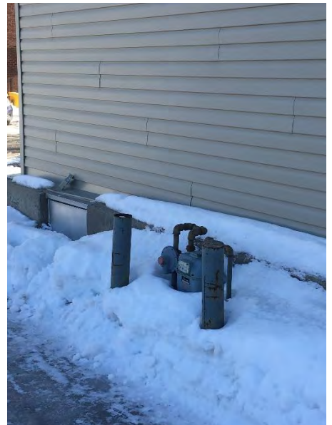
Gas connection & meter (east)
