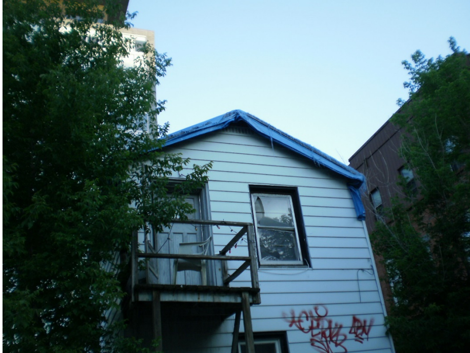
Photo 5 – Tarps to prevent wildlife access to the remaining residence in the southwest portion of the site. View looking south to the north portion of the residence
