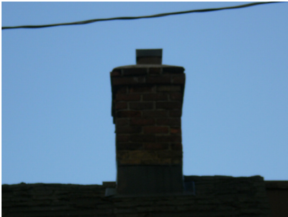
Photo 4 –Chimney on the remaining residence in the southwest portion of the site.
