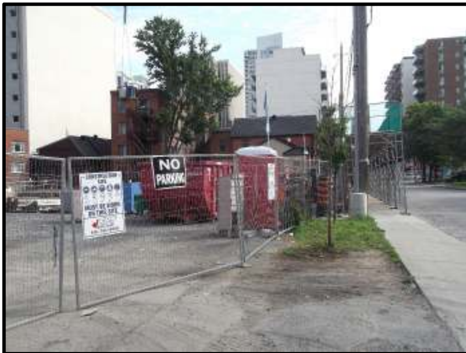
Photograph 4: View of southeastern portion of Phase I Property, facing east. Photograph illustrates use of a portion of 307 Lisgar Street and 293 Lisgar Street as a staging area for the residential construction on the adjacent property to the east (287 Lisgar Street).
