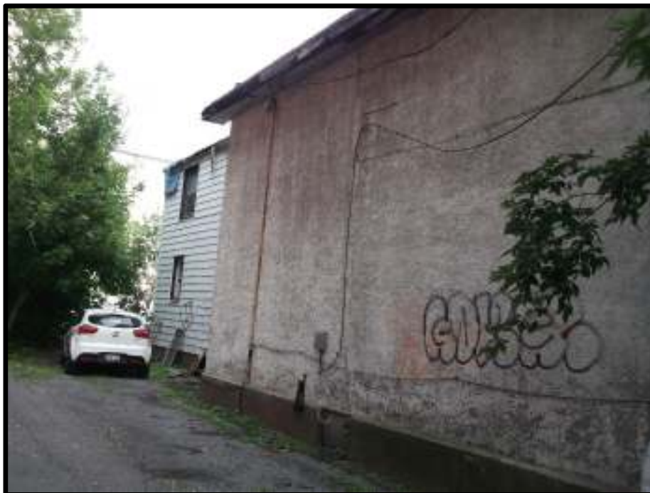
Photograph 2: View of west face of 309 Lisgar Street, facing northeast. Vent and fill pipes can be seen exiting the foundation of the original portion of the building structure.
