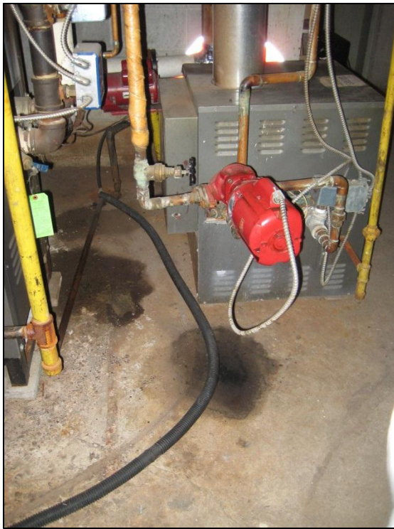
Photo No.15: View of the stained areas on the furnace room floor
