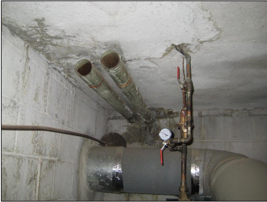
Photo No.17: View of suspected old fuel oil fill and vent pipes in the furnace room.
