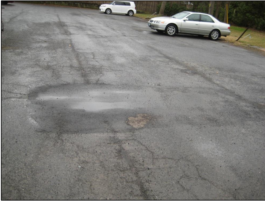
Photo No.7: View of asphalt cut area in the central section of parking lot (facing south)
