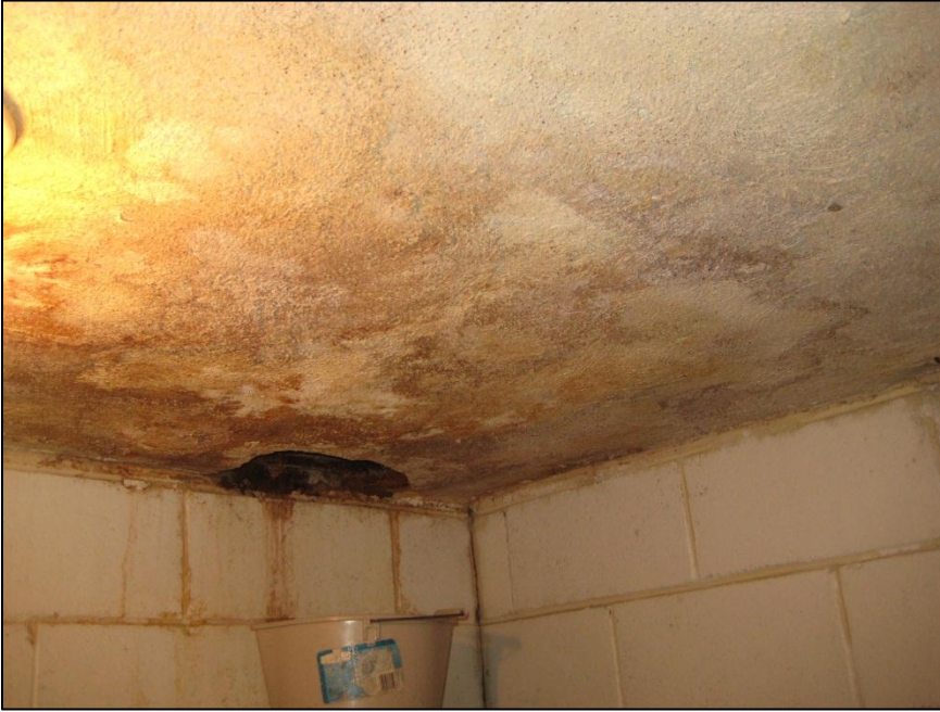
Photo No.19: View of water damaged ceiling in a storage room
