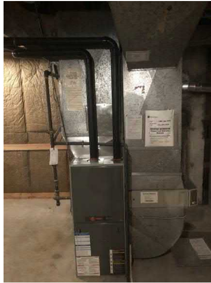
Photo 16: Furnace in basement of 810 Vick.
