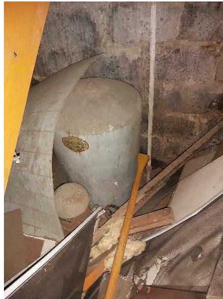
Picture 1: Water tank in basement of 2830 Carling.
