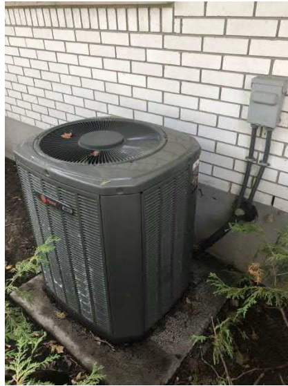
Photo 21: Air conditioning unit at the front exterior of 810 Vick.
