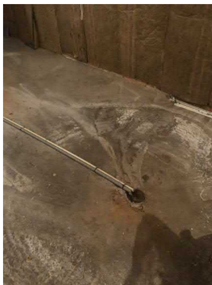
Photo 15: Basement drain in 810 Vick.
