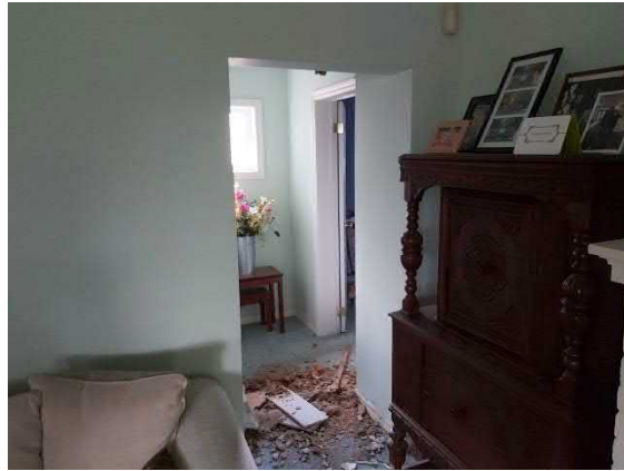
Photo 7: Damaged ceiling with mould above on the main floor of 2830 Carling.
