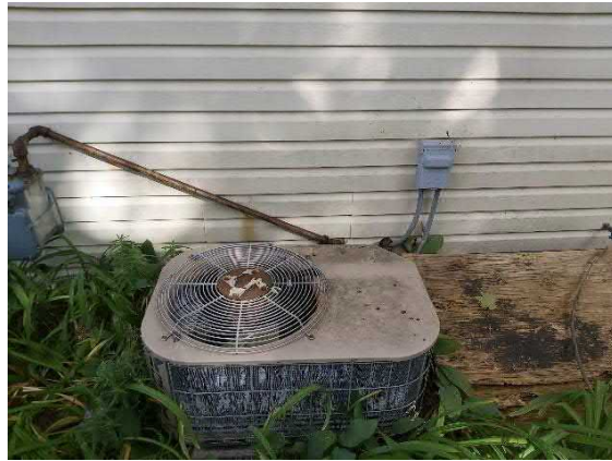
Photo 9: Air conditioning unit at the front exterior of 2830 Carling.
