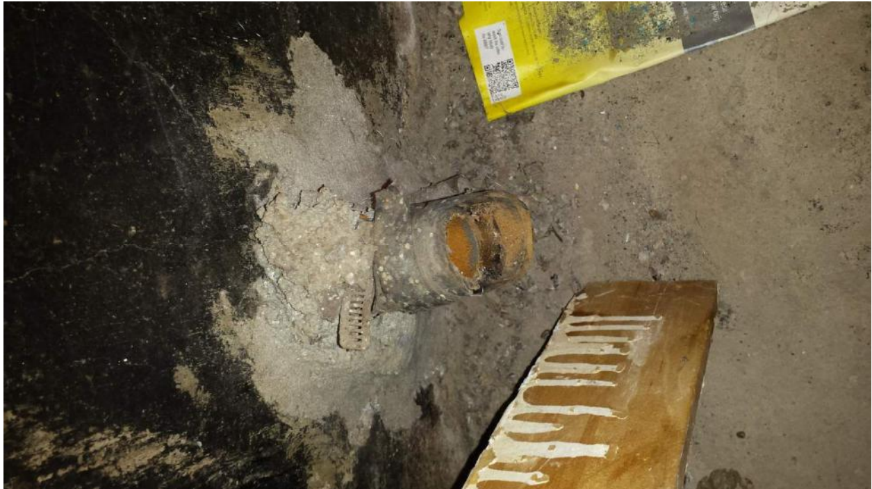
Photograph 5: Exposed pipe and possible asbestos-containing material in the basement level of 3835 Innes Road.
