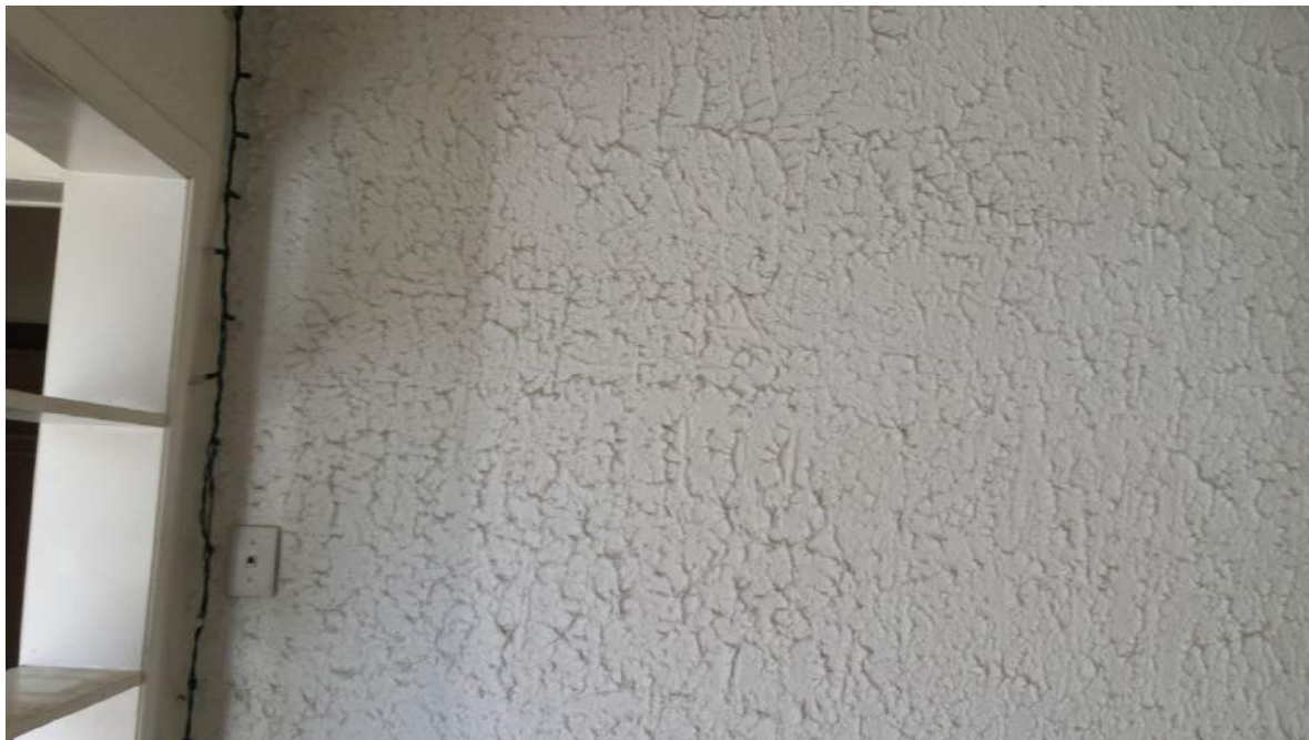
Photograph 8: Interior wall at 3843 Innes Road, finished with a potential asbestos-containing plaster material.
