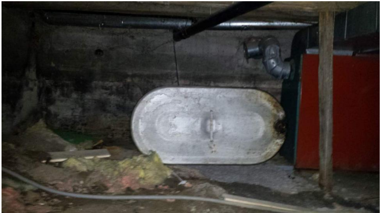
Photograph 12: Aboveground storage tank and furnace (at right) in the basement at 3843 Innes Road.
