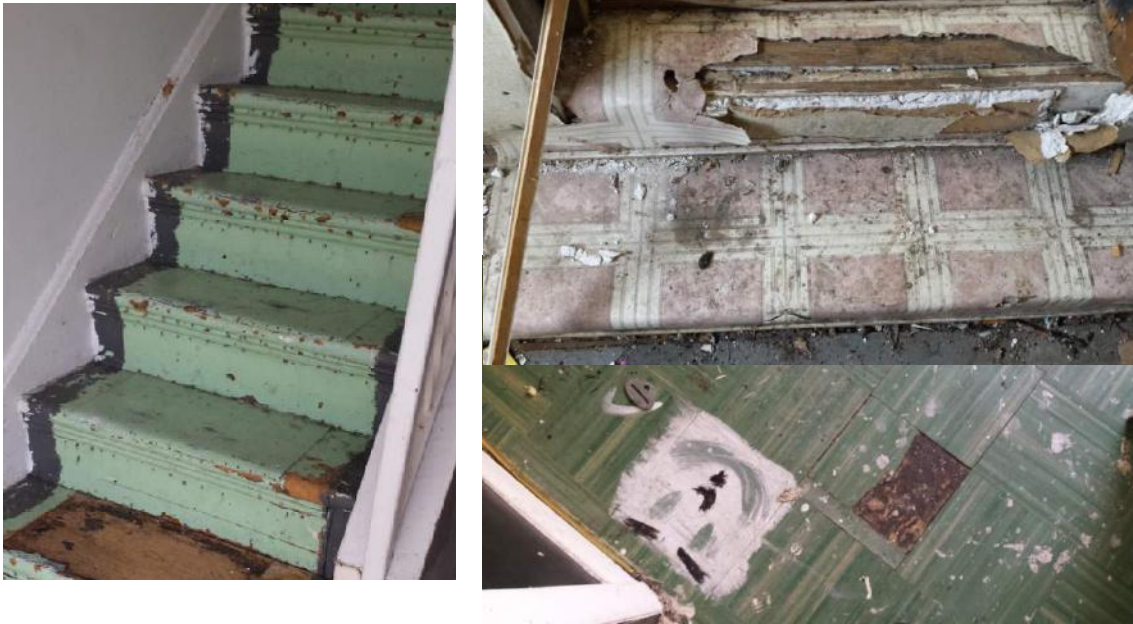
Photograph 9, 10 and 11: Possible asbestos-containing flooring materials at 3843 Innes Road, in poor condition.
