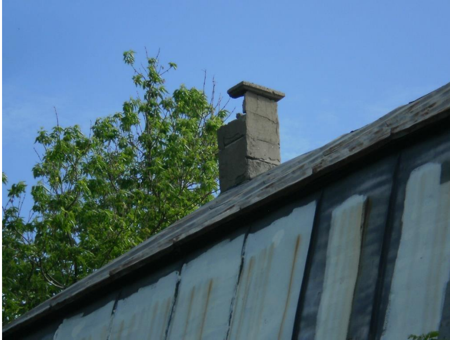
Photo 7 – Concrete chimney on the residence in the northeast portion of the site is in poor condition and open. View looking east
