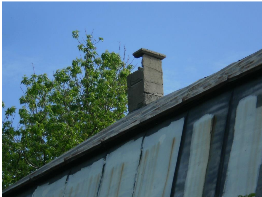
Photo 7 – Concrete chimney on the residence in the northeast portion of the site is in poor condition and open. View looking east
