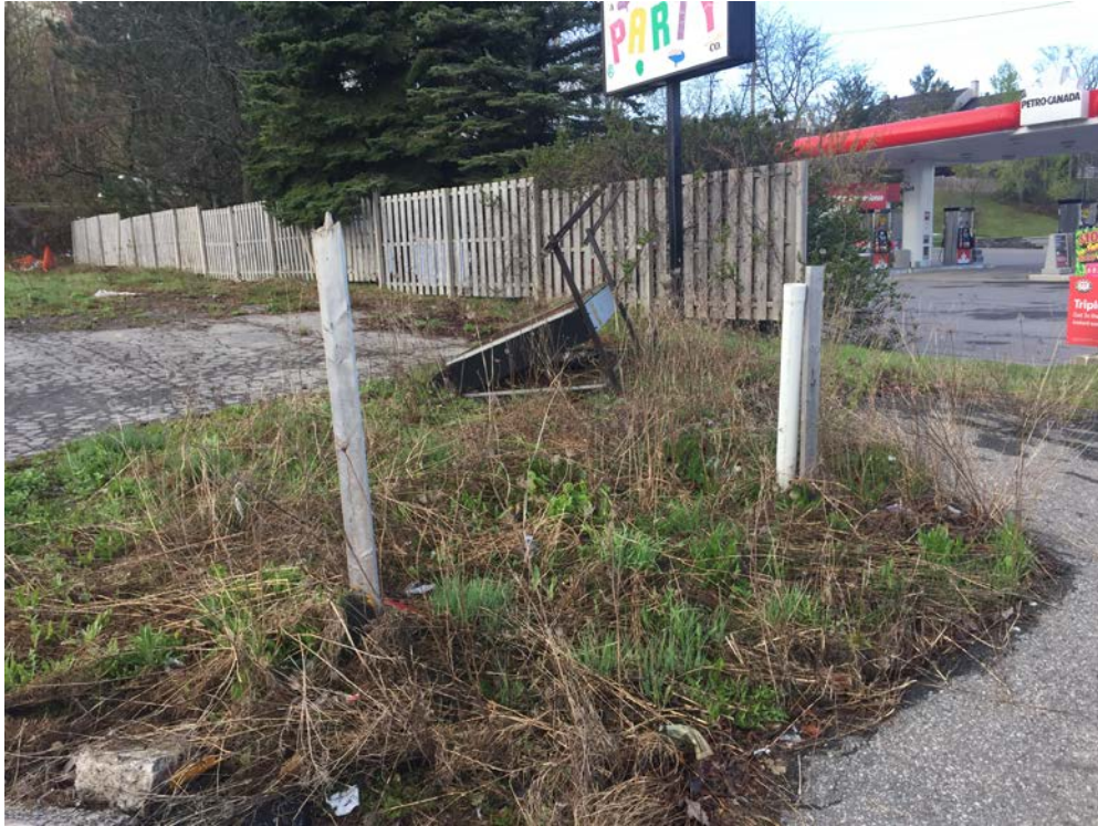
View of some buried utilities located in the north side of the site.
