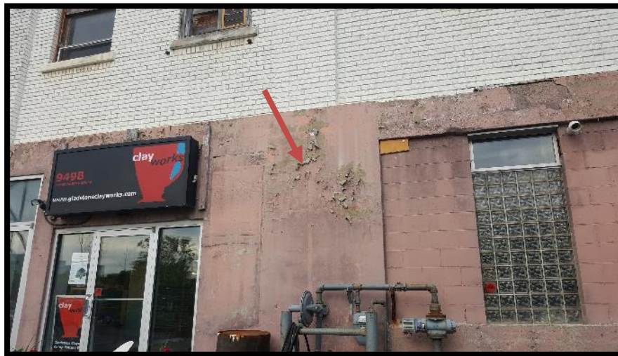
Photograph 8 – View of peeling paint (see arrow) on the exterior of the Site building associated with 951 Gladstone Avenue.
