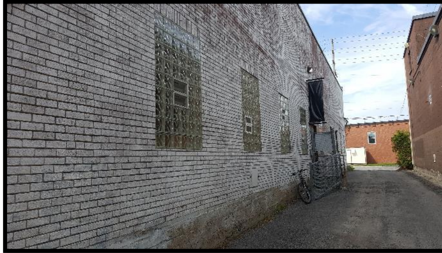
Photograph 1 – View of a portion of the north elevation of the Site building associated with 951 Gladstone Avenue.
