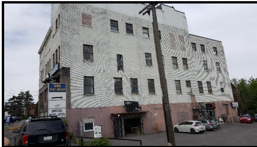
Photograph 2 – View of a portion of the east elevation of the Site building associated with 951 Gladstone Avenue.
